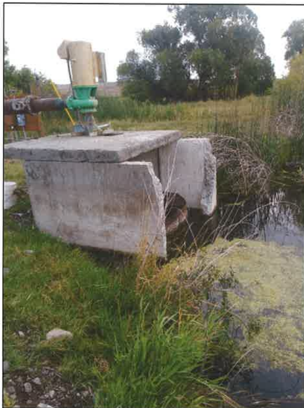
The pump which supplies water to the pivot.
