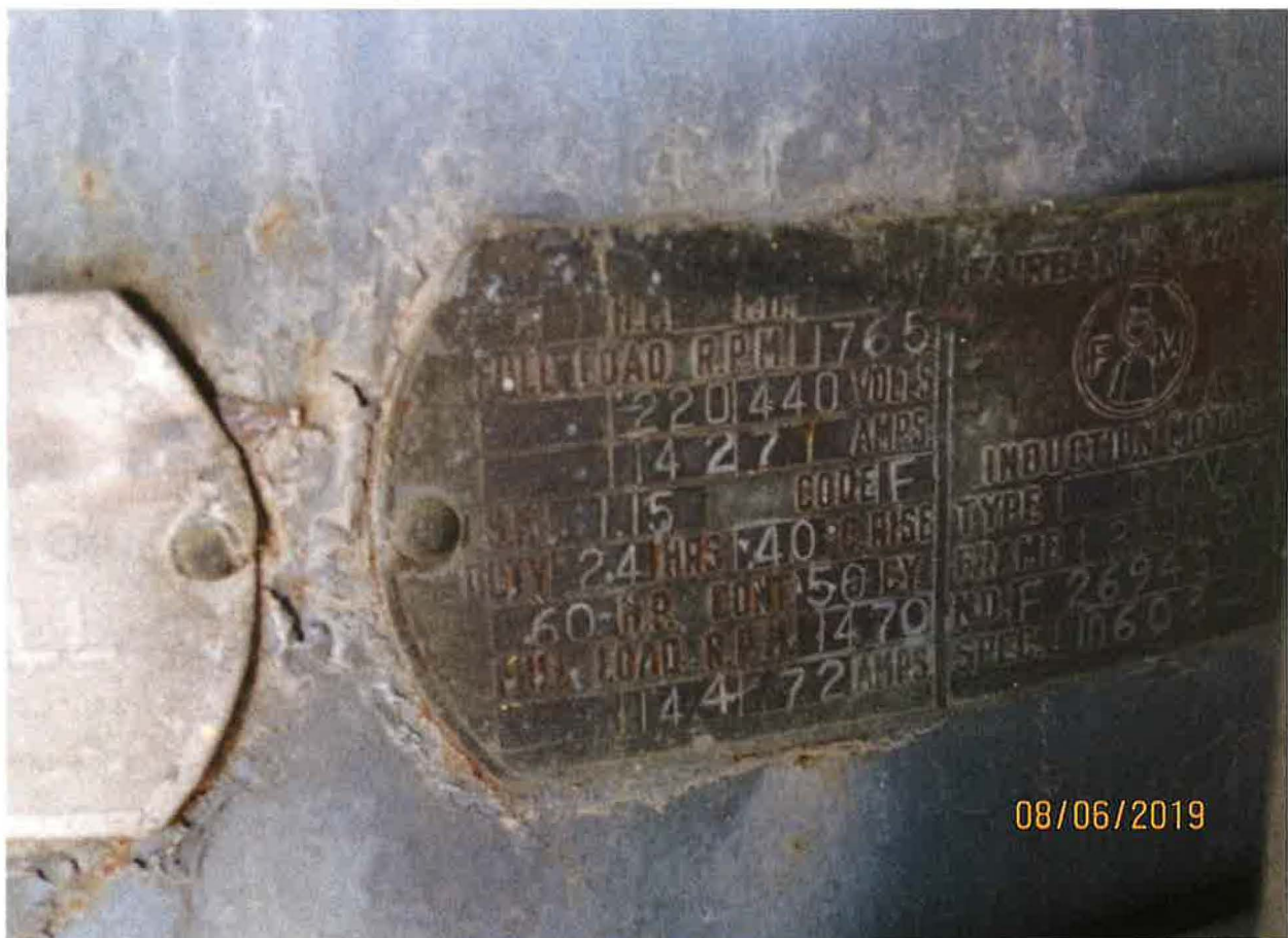
Pump tag showing 60HP pump.
