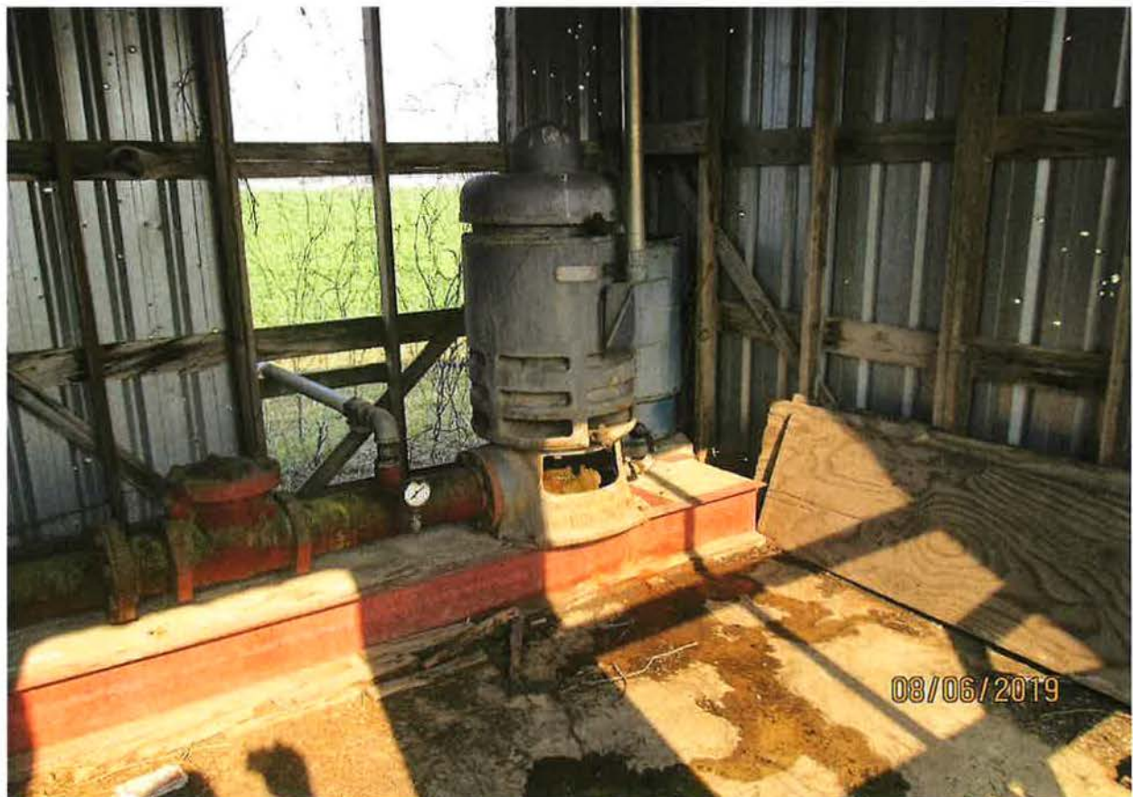
Well and pump.
