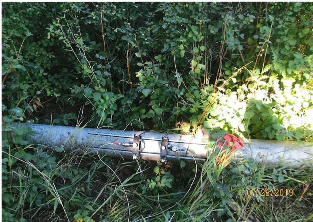
Aluminum pipe mainline where measurement was performed used GE Panemetric Flowmeter. Flow was measured at 266.9 gpm or 0.59 cfs.
