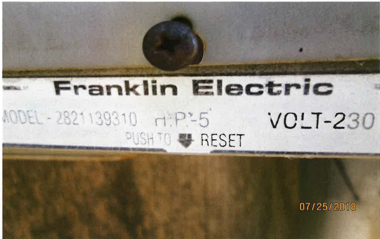
5hp pump from lake to storage tank 415 feet up hillside.
