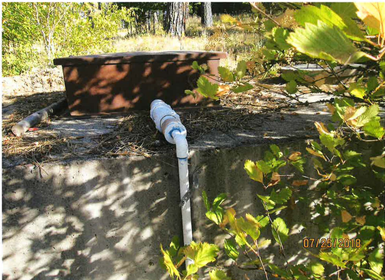
3,000 gallon storage tank with gravity fed system to homes.
