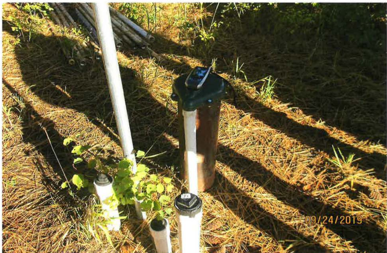
Well D0054667 with 5hp pump.
