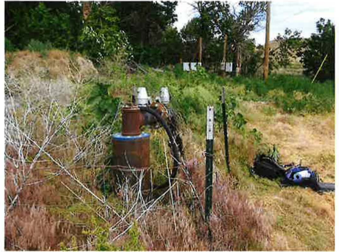
Facing North. The control panels for the pump for the well and the pump from the pond are in the background.
