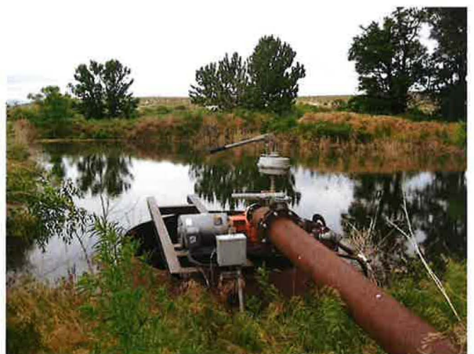
Facing South. Pump from the pond. Surface water diverted from Pickett Creek (Water Right 57-53) enters the pond from the west (right side of the photo).
