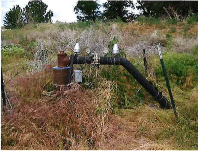
Facing west. The berm separating the pond and the well is immediately behind the well. Mounting brackets for the flowmeter are in place on the right.
