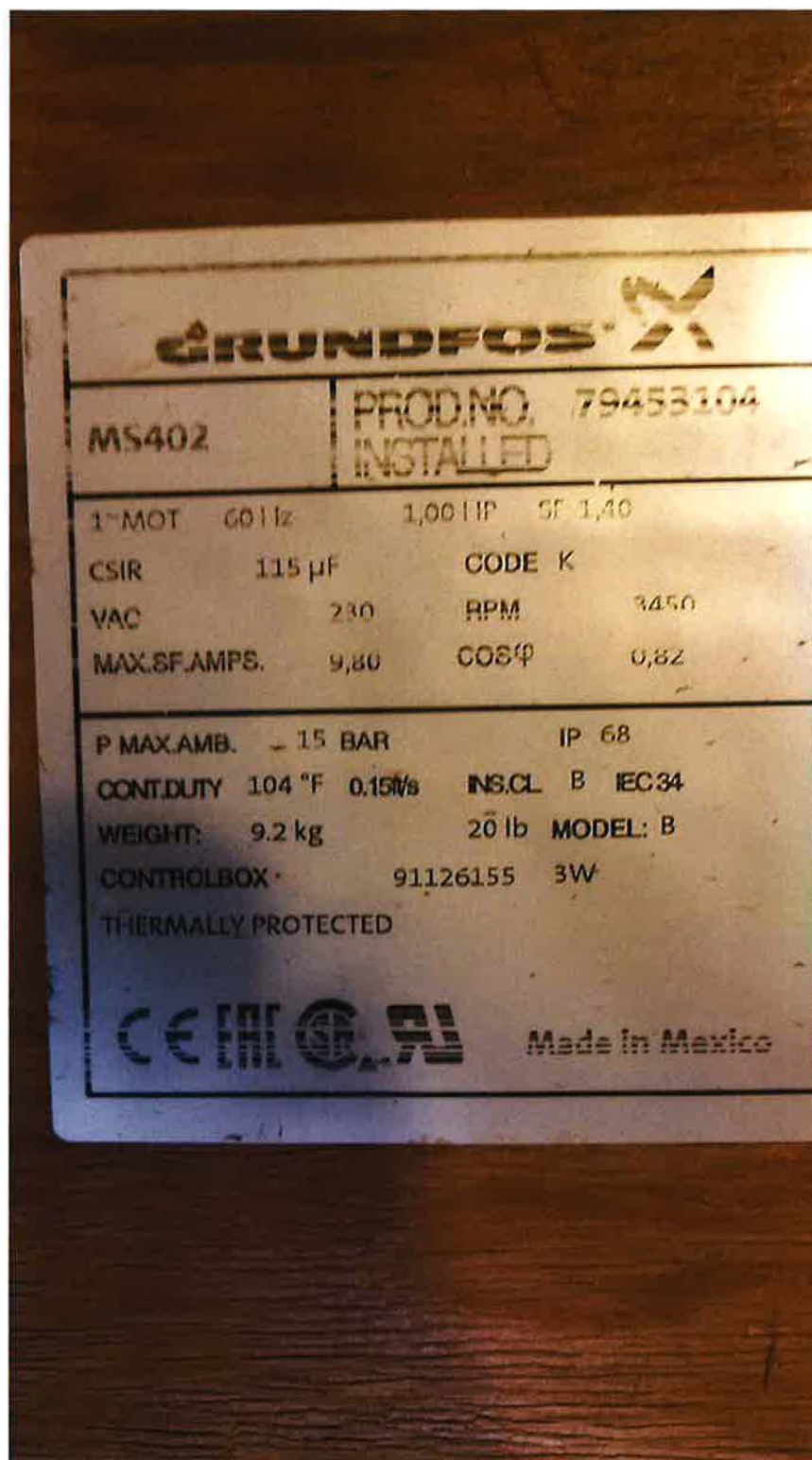
Photo #2 – Pump Nameplate
