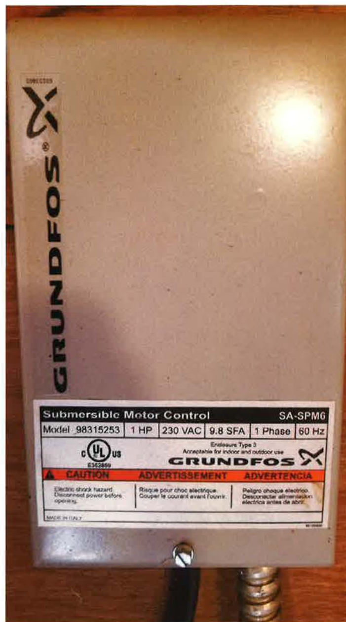
Photo #3 – Motor Nameplate
