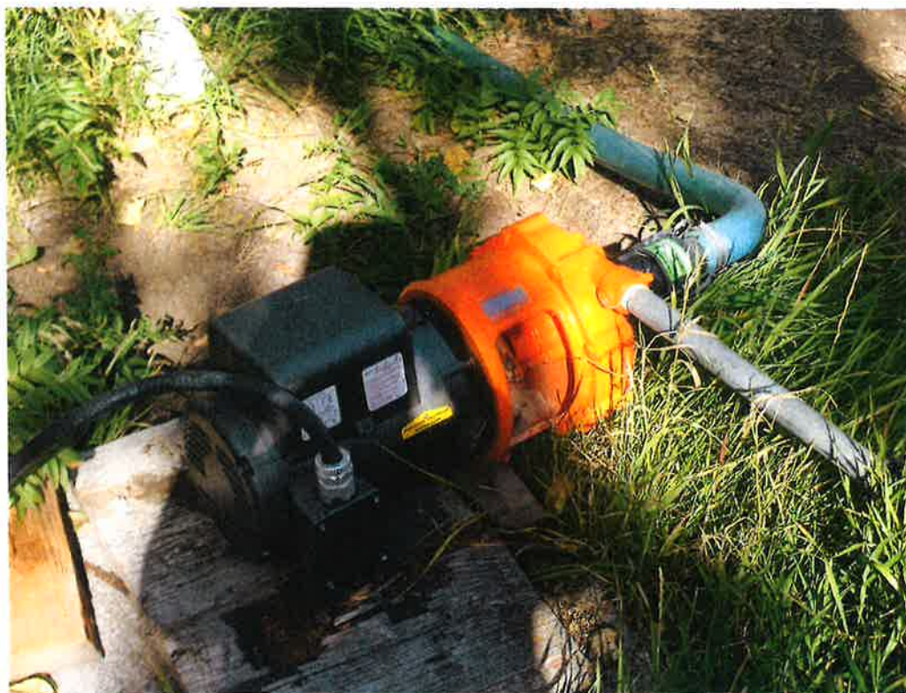
5 HP pump on the river bank
