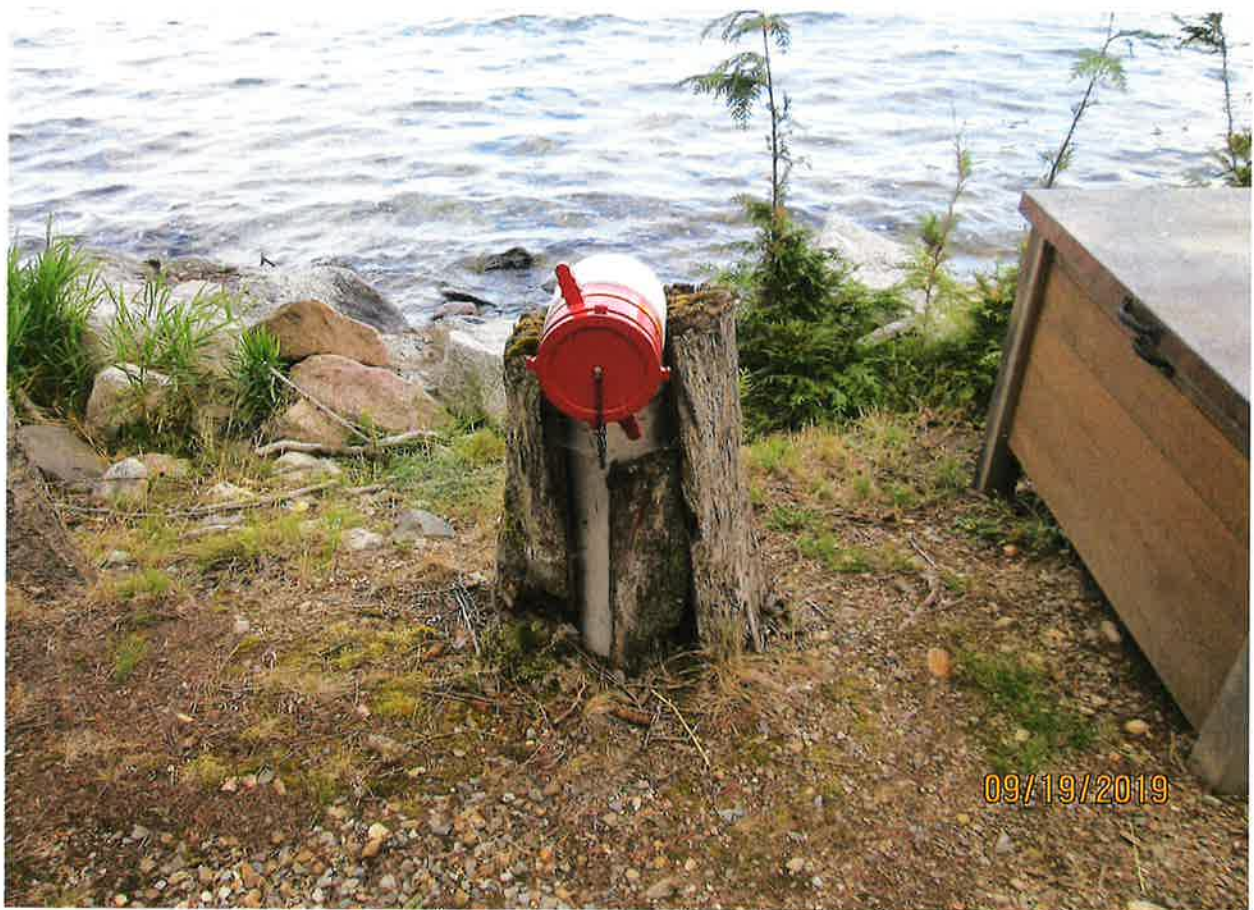
"Dry" fire hydrant made with 6 inch piping.
