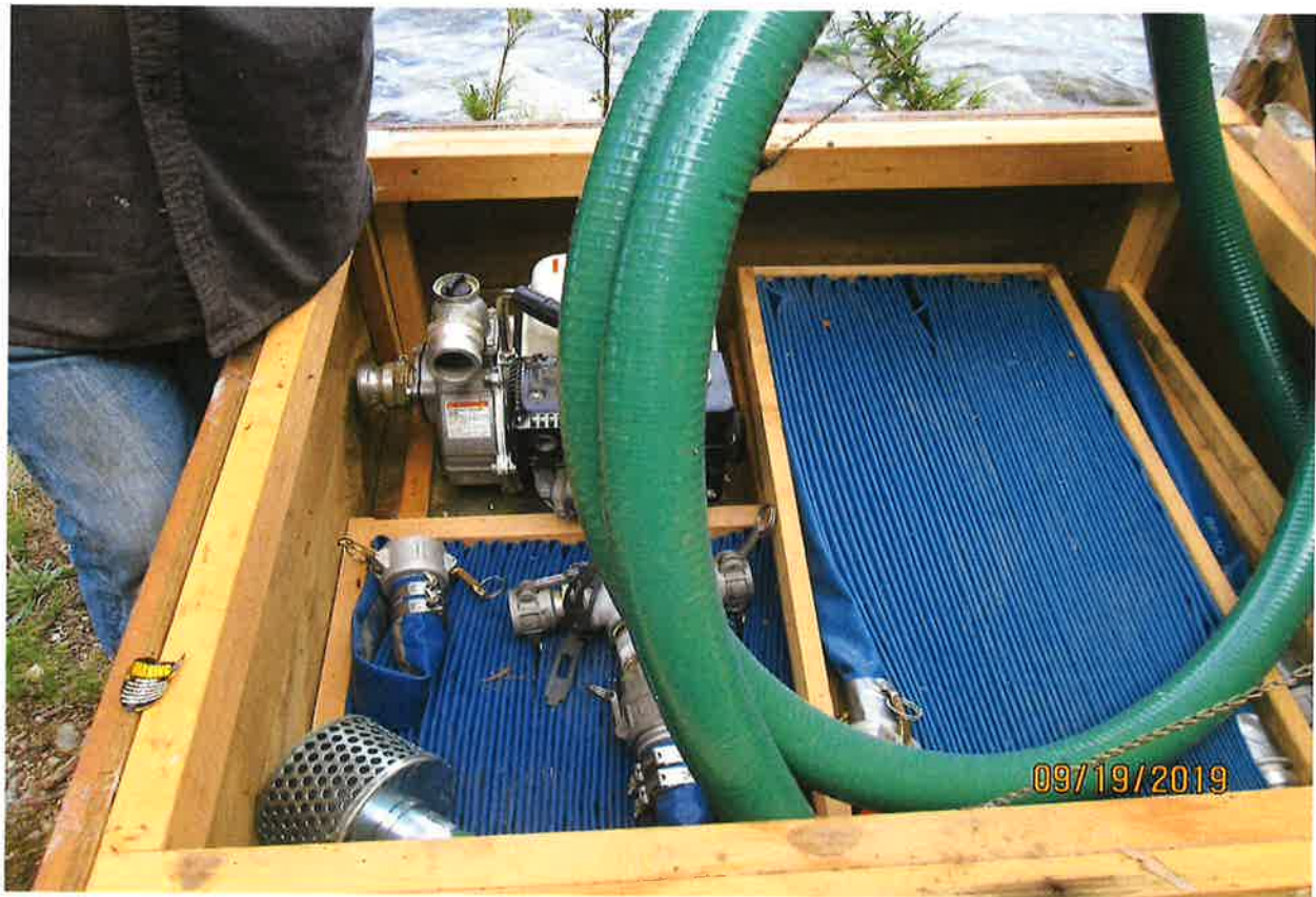
Applicant also had emergency fire protection station located next to dry hydrant in case of emergencies.
