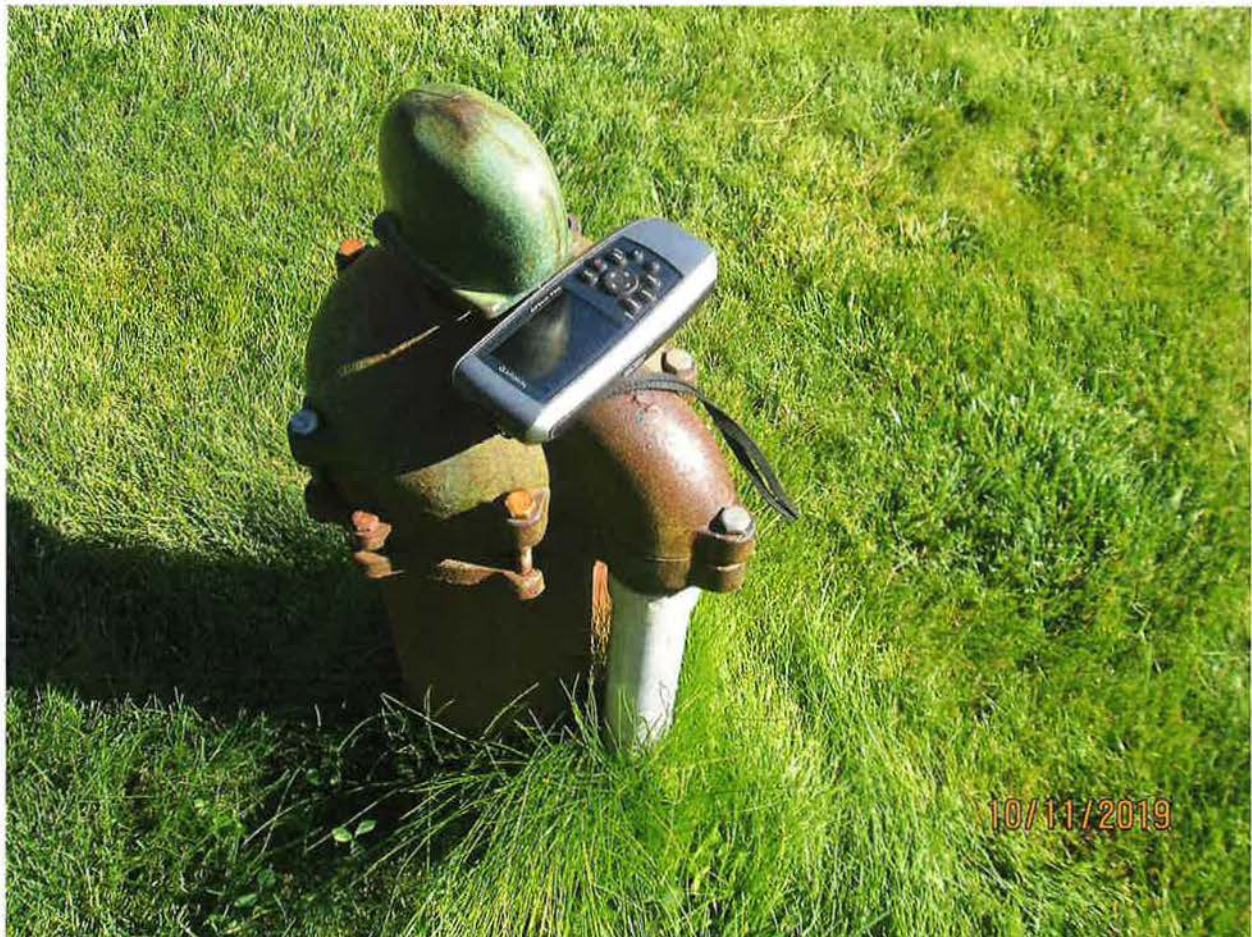
Well 95-93-N-169-000 with 3hp pump.
