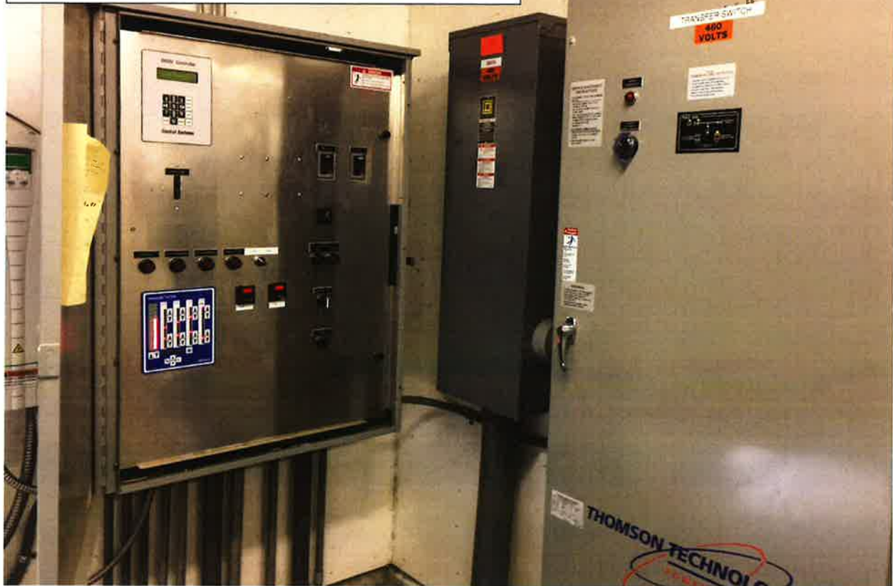
Pump 3 (100 hp) panel and pump system PLC on left, automatic transfer switch for backup generator on right
