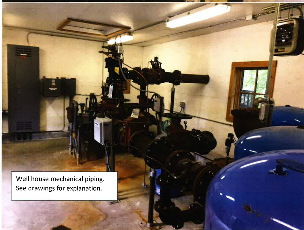
Well 2 with junction box and discharge pipe for pump 1 (15 hp) in foreground and left; discharge pipe and junction box for pump 3 (100 hp) in back
