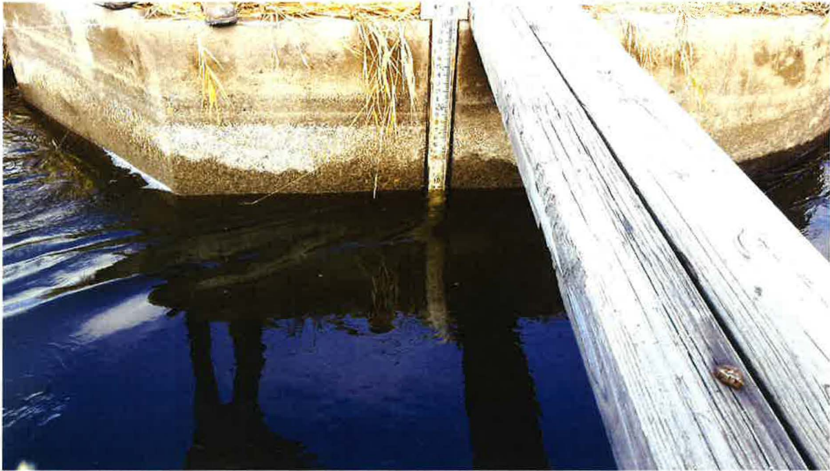
Ramped flume measurement device and staff gage at point of diversion
