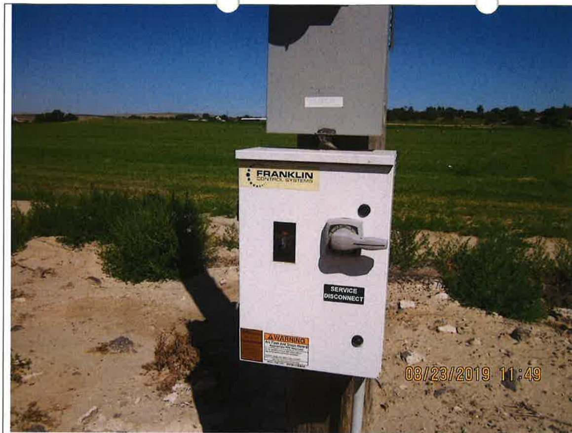
Figure 5. Franklin control panel.
