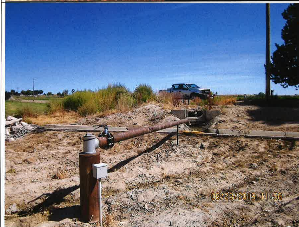
Figure 2. Well head with open discharge pipe into ditch.
