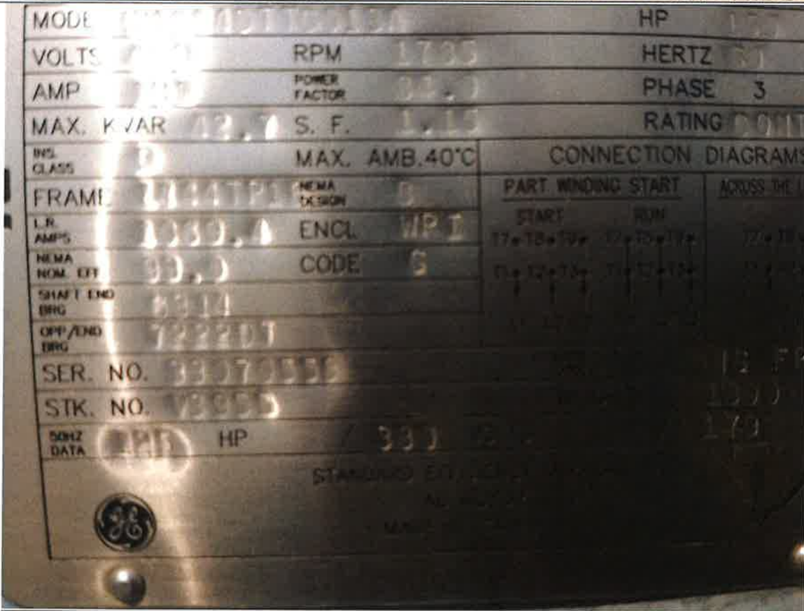
Figure 4. Pump label from well #2 showing a 150 hp pump.
