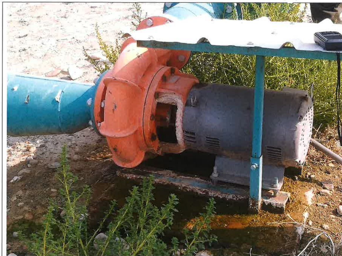
Figure 7. 15 hp booster pump to pivot located part way uphill.
