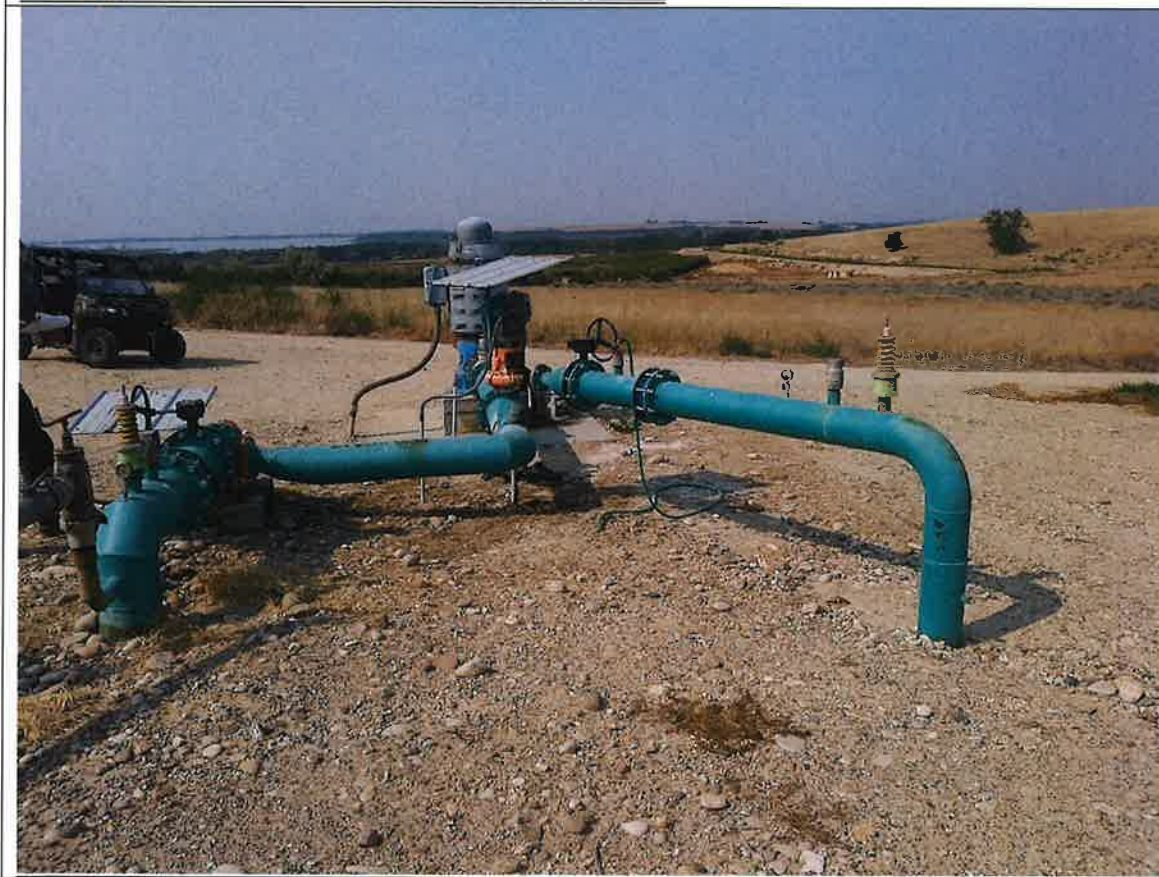
Figure 6. Well #2 with 150 hp vertical turbine pump and centrifugal booster pumps feeding two mainlines.
