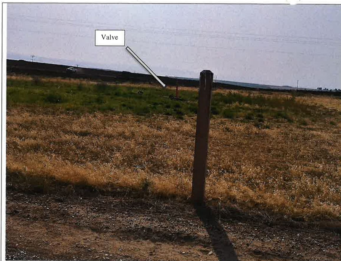
Figure 11. Photo of valve and pipeline in the long narrow pasture west of driveway. Irrigation infrastructure is in place however the pasture sparsely irrigated.
