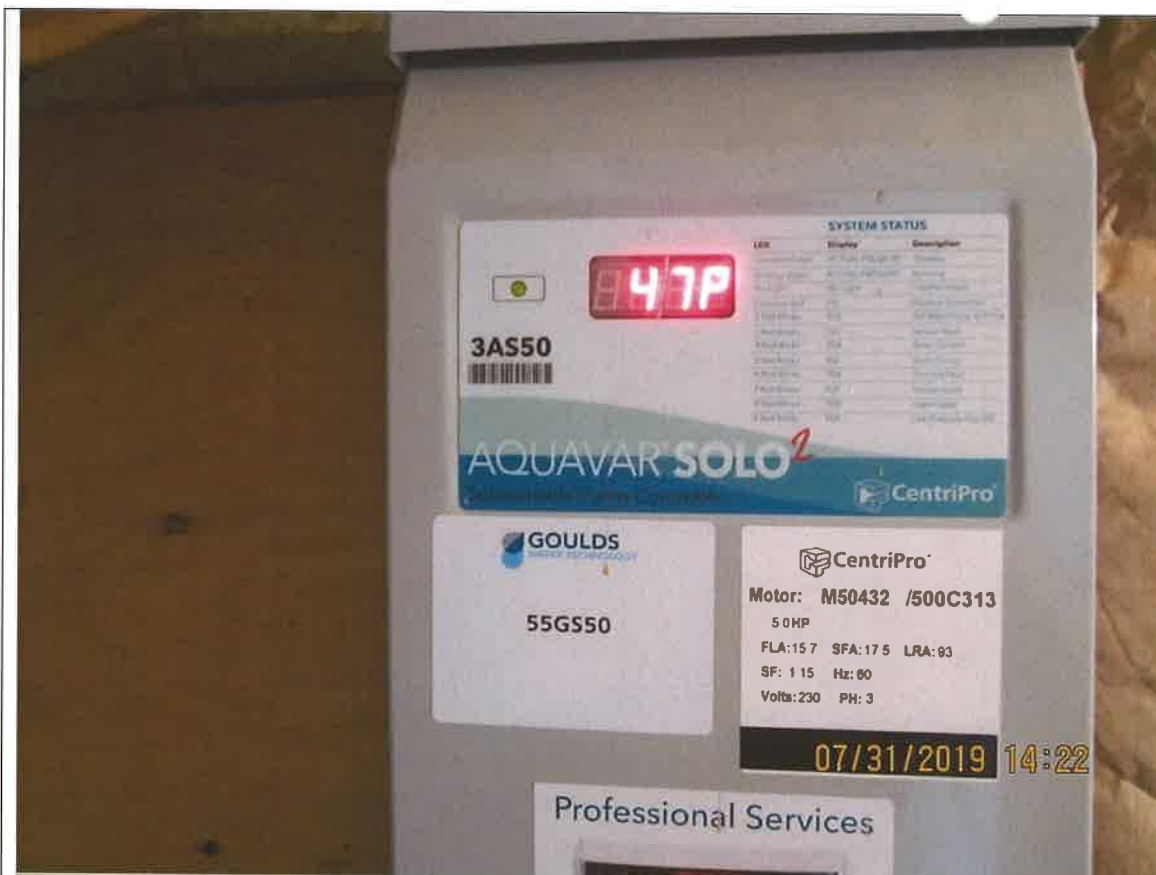
Figure 3. Aquavar Solo 2 VFD pump controller, digital display showing 47 psi.
