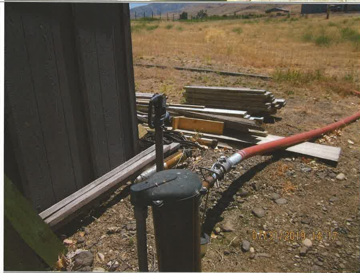
Figure 2. Well head with hose going to mainline.
