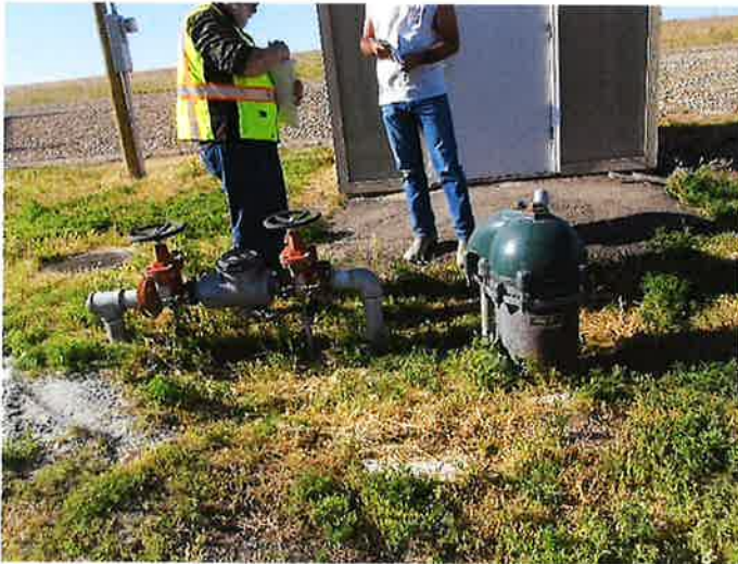
Well, well house and valves to each property irrigation system. South end facing south next to Lewis Lane.
