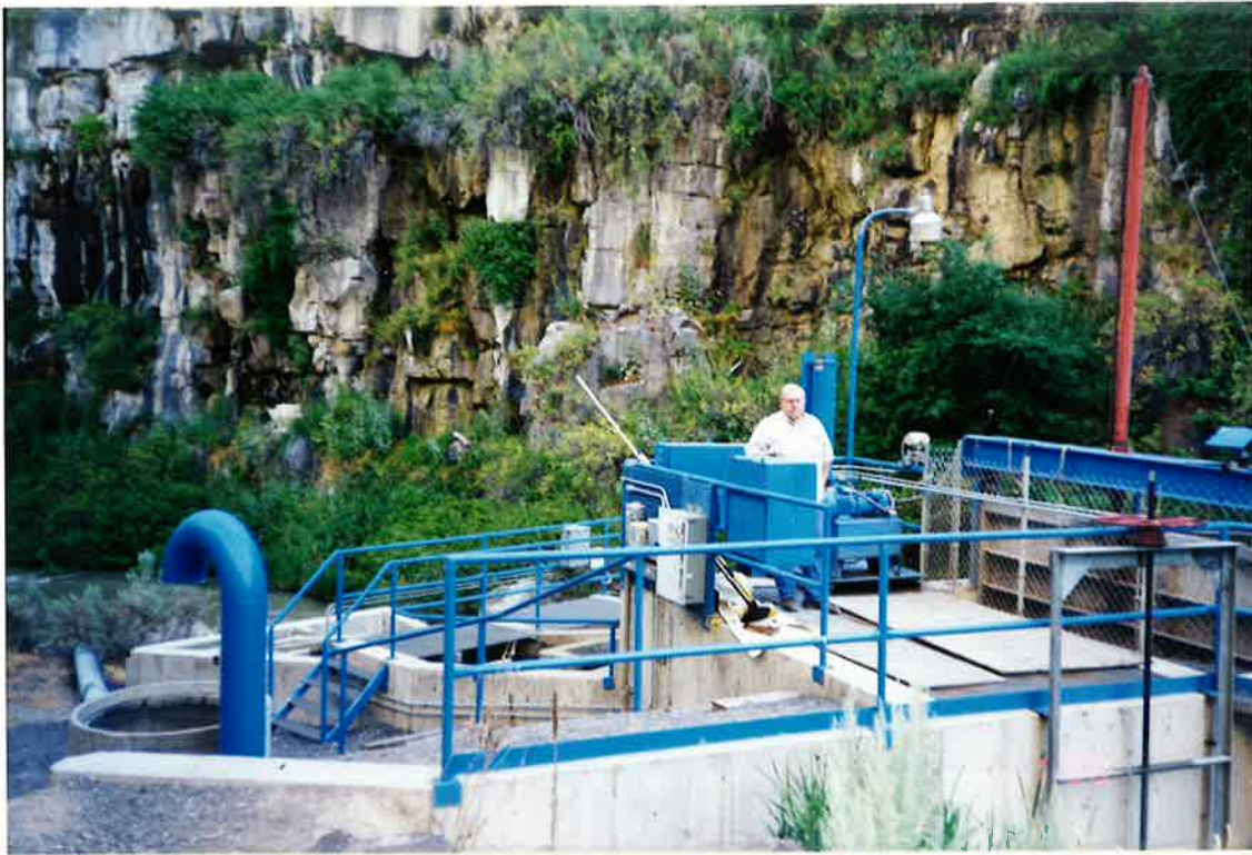
Controlling Mechanism At POD; Pipeline Inlet ↗
