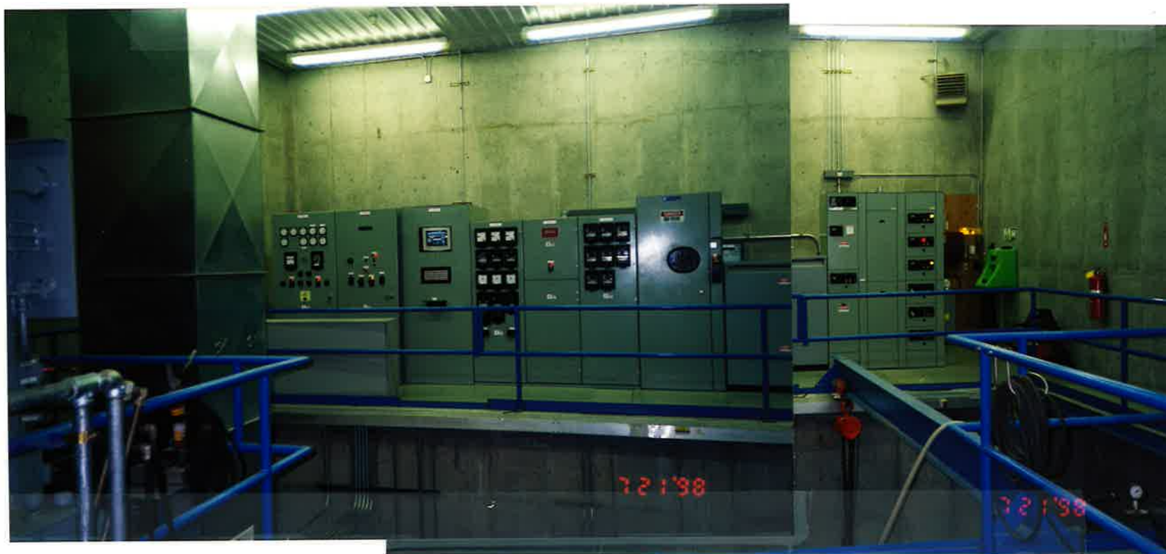
Interior of Power Plant
