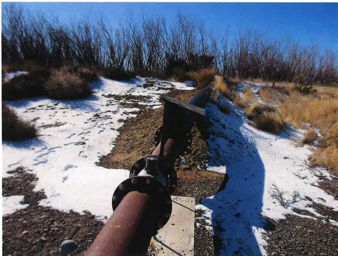
Pipe from well to pond. Note flowmeter in lower center of photo.
