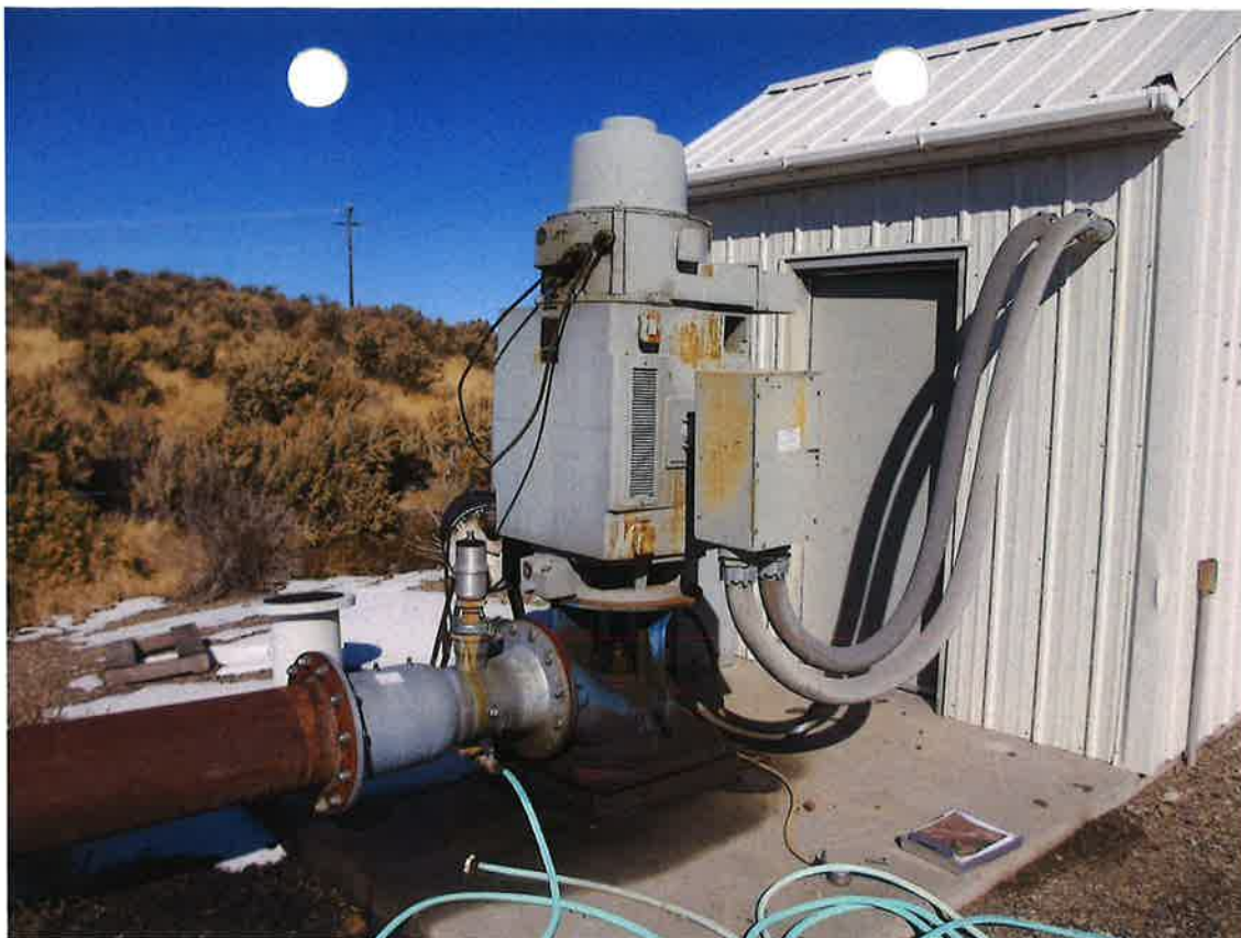
Well and pump house.
