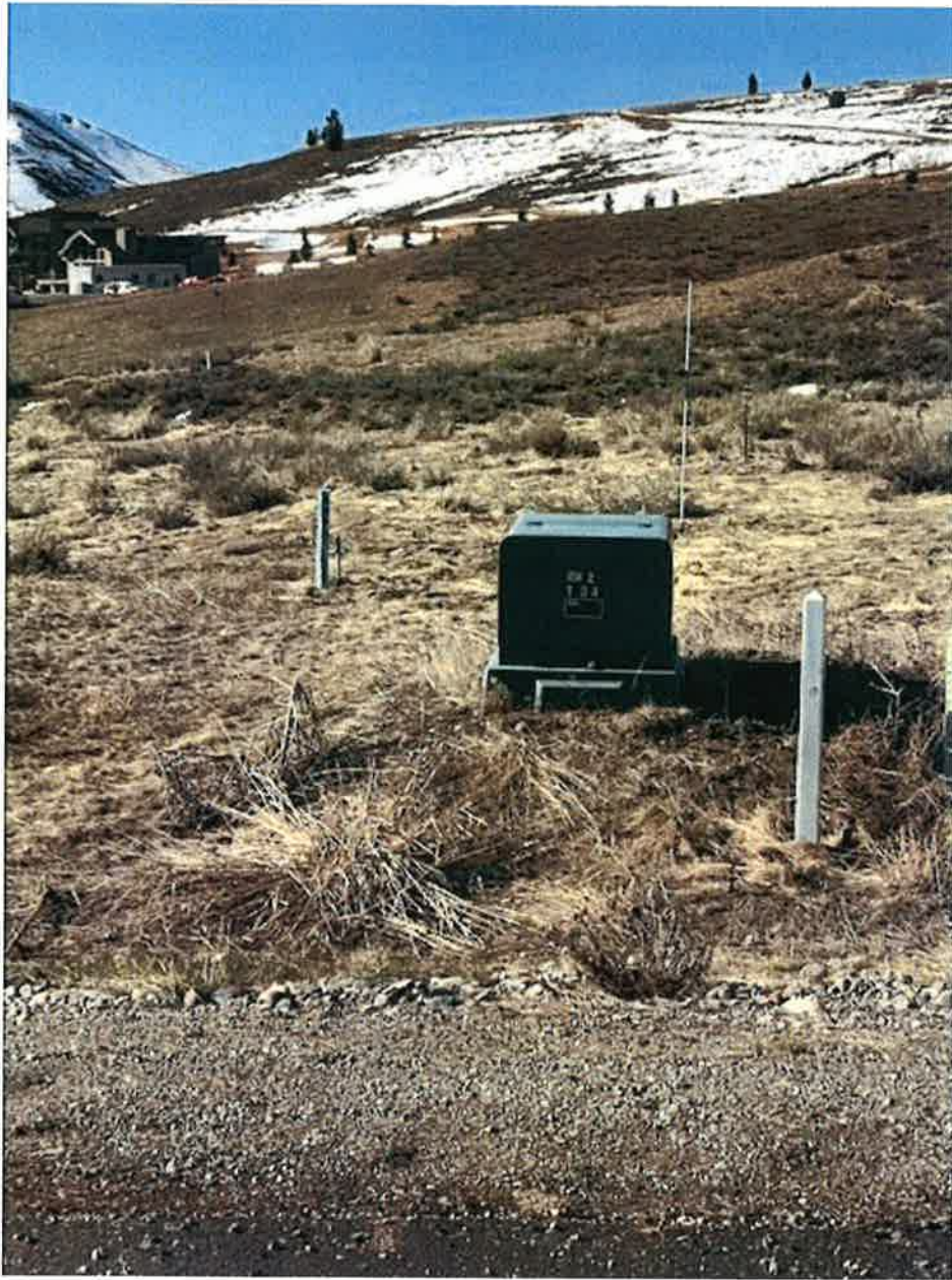
Example of stubbed in service line
