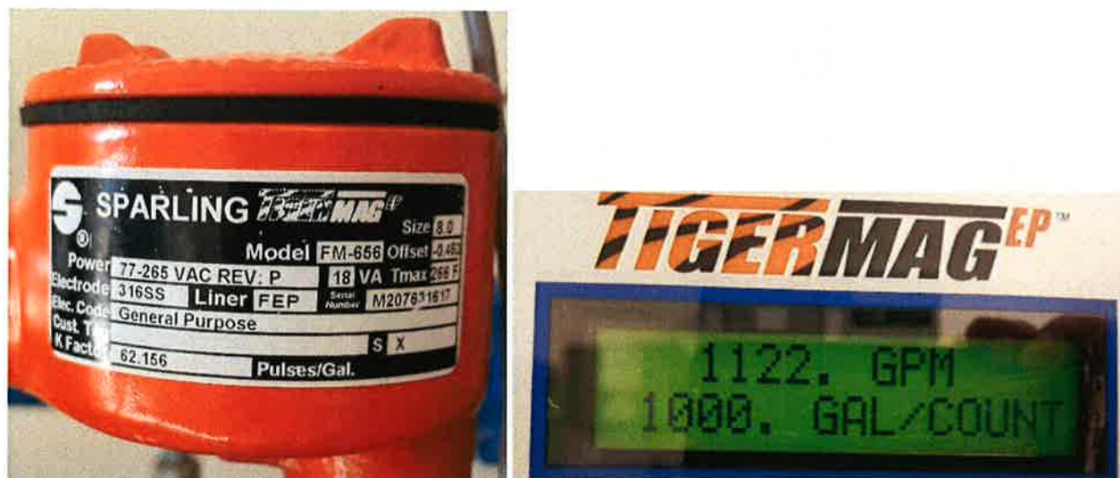
Meter and meter readout
