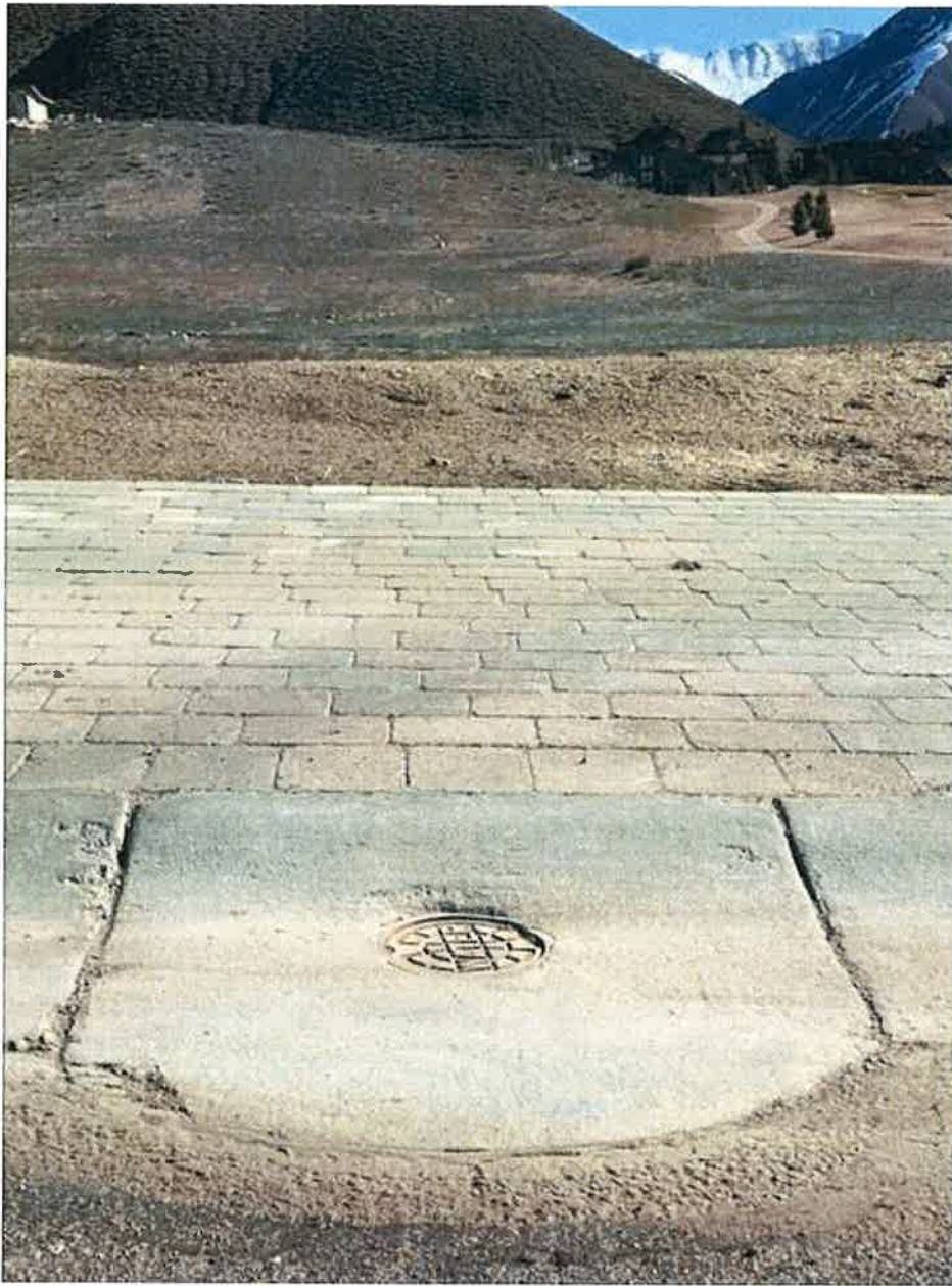
Example of stubbed in service main
