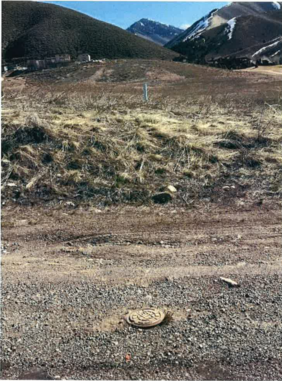
Example of stubbed in service main
