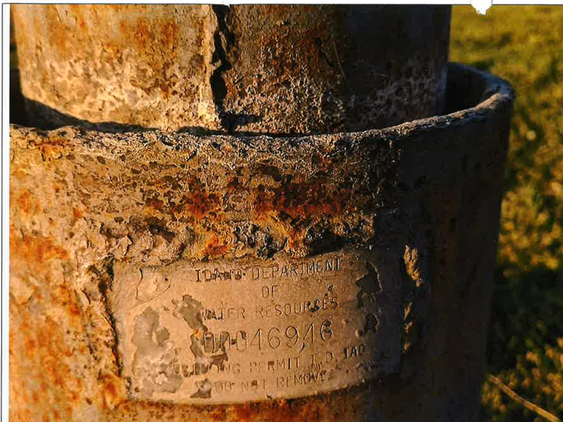
Figure 1. Well tag on bottom casing, #D0046946.
