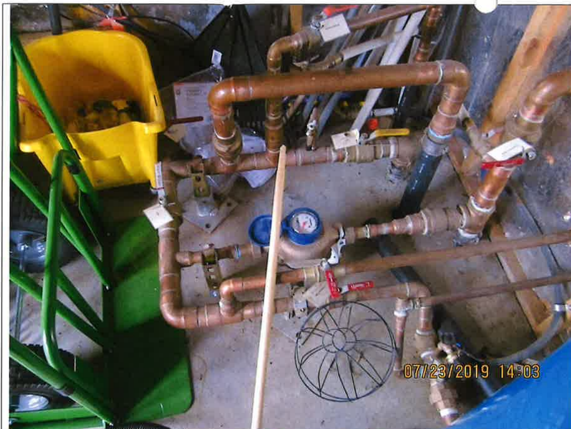
Figure 5. Inside the pumphouse.
