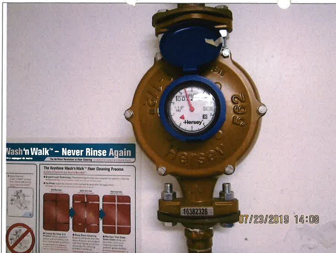
Figure 15. Lodge kitchen meter.
