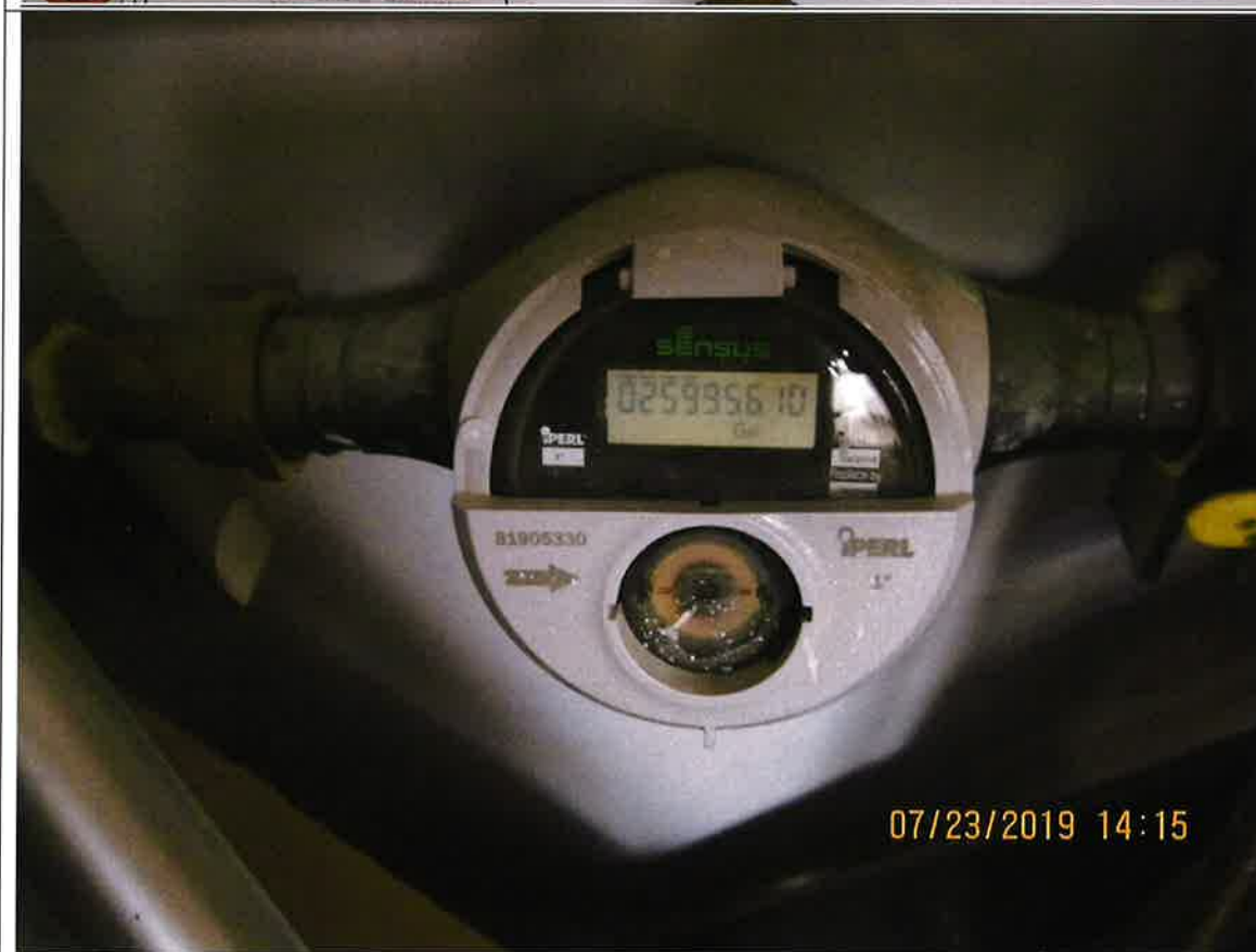
Figure 16. Farmhouse basement meter.
