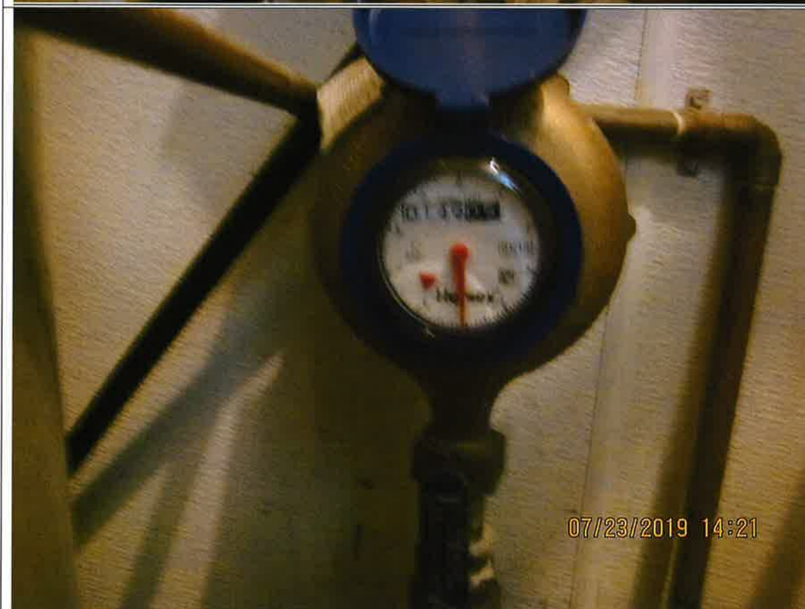
Figure 18. School house meter.
