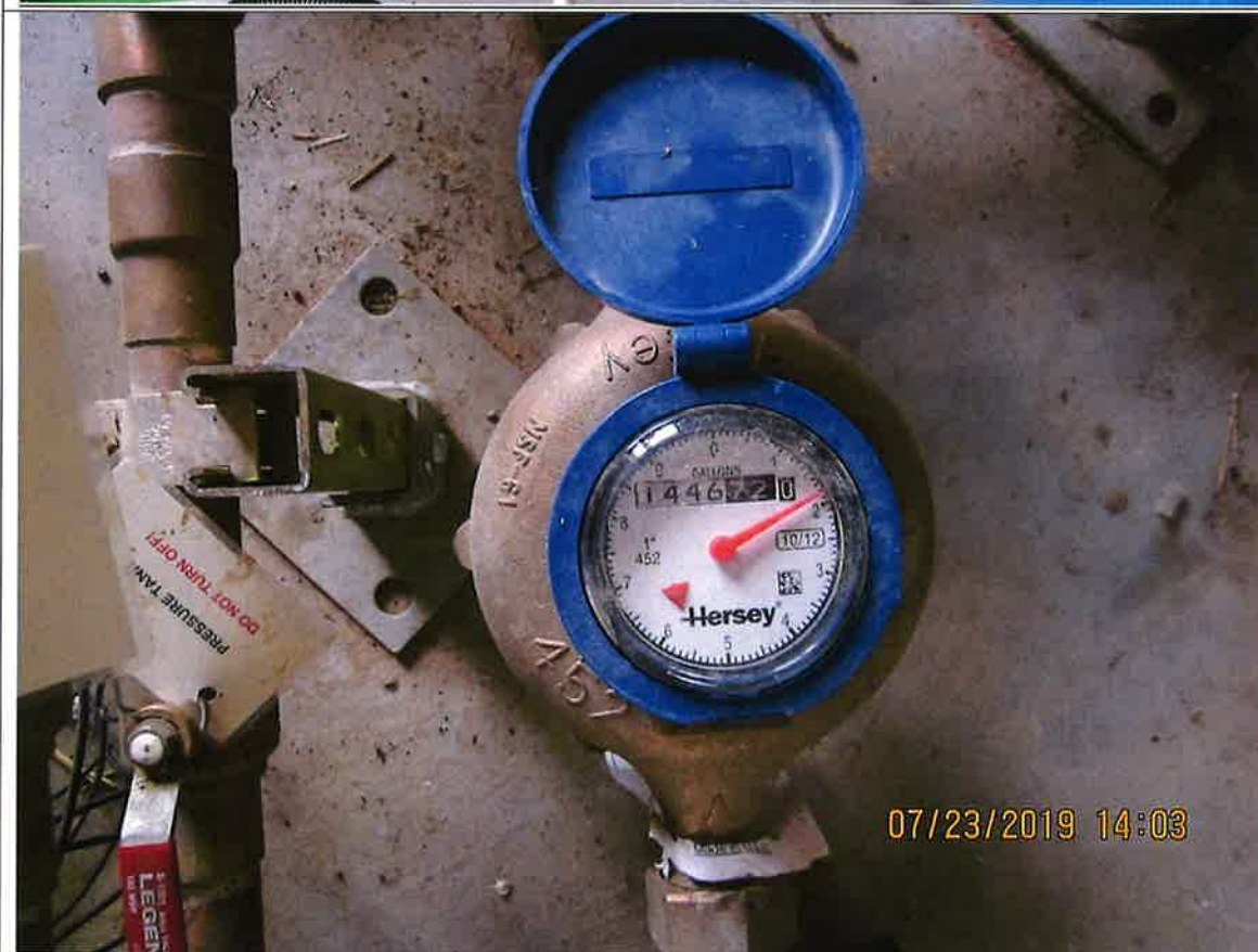
Figure 6. Pump house flow meter.
