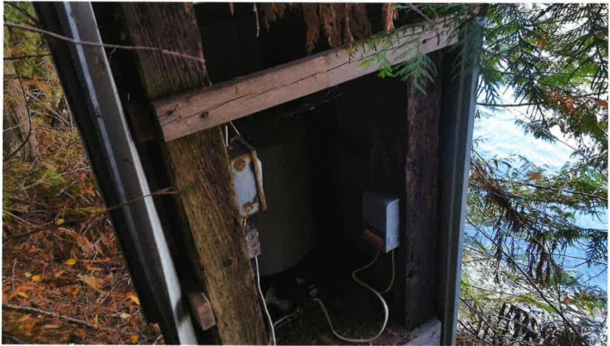
Wiring for Pump house that diverts from Spirit Lake.
