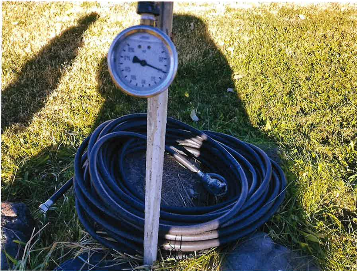
Looking at irrigation spigot #2 in front yard of the house. Test yielded 40 psi.
