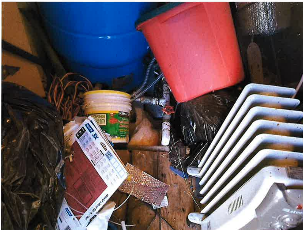
Looking inside pump house at pressure tank. Note pressure gauge has been removed due to a leak.
