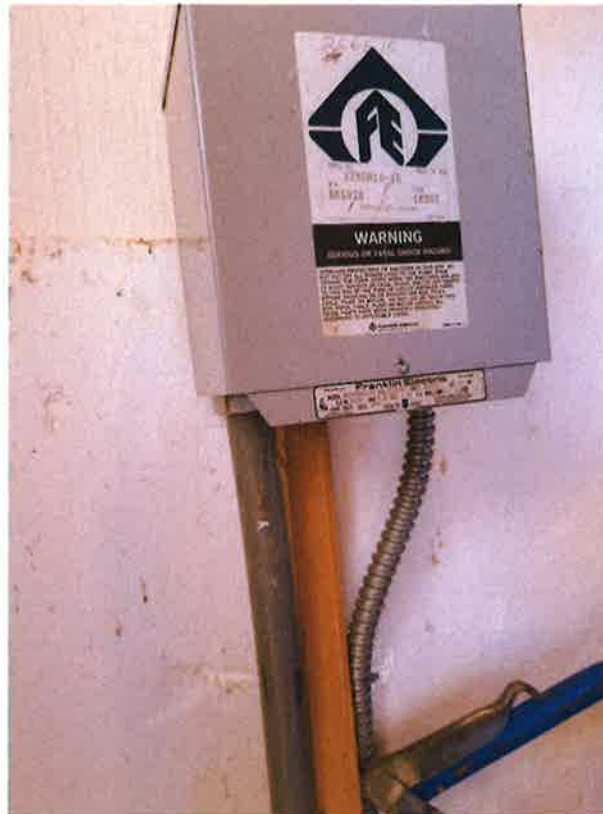
Looking inside pump house at power supply box to well (1.5 HP submersible Berkeley pump)
