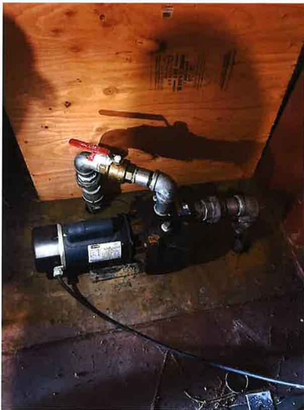
Pump inside container. Input from well on right, output on left.
