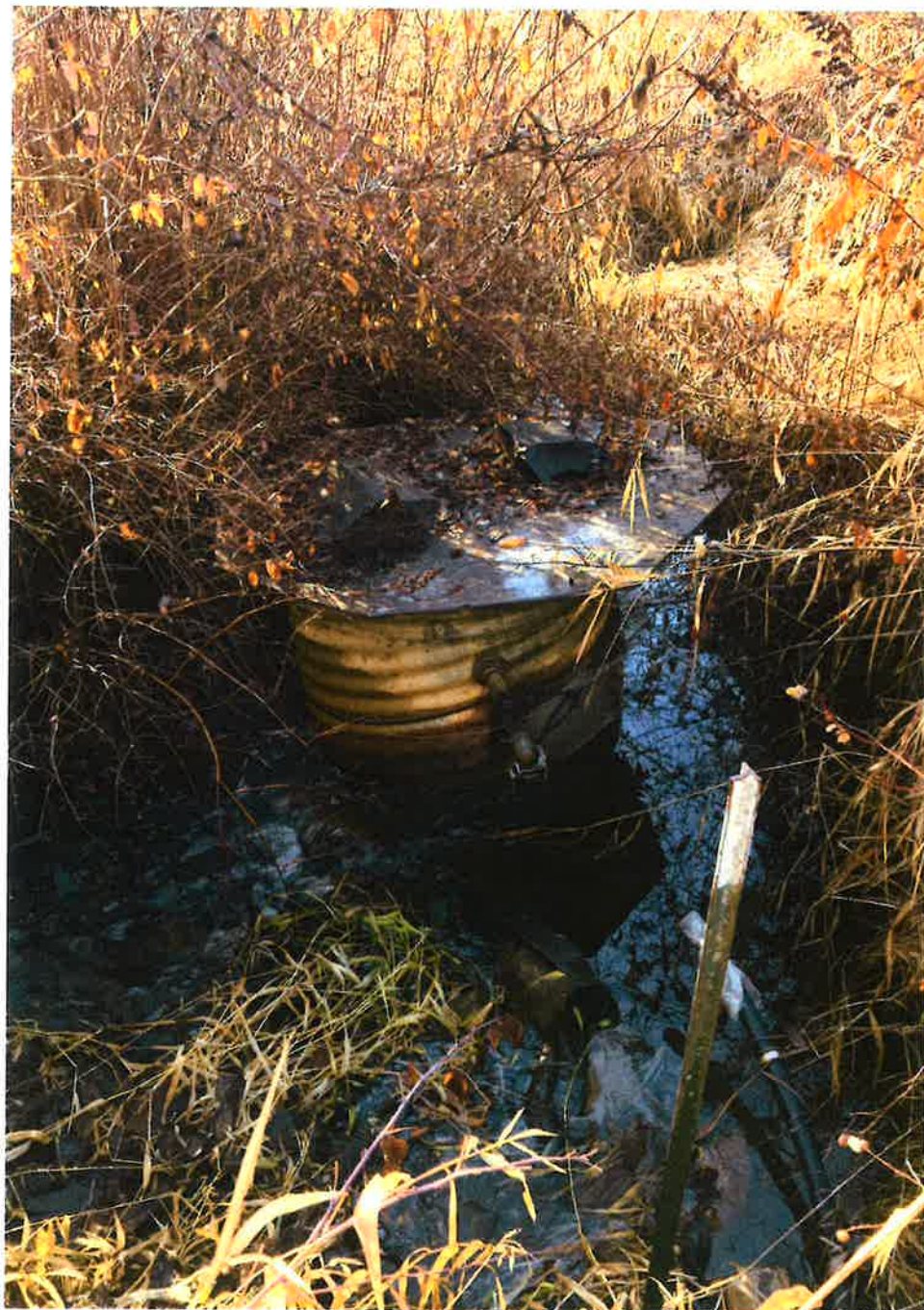
Lawn irrigation intake.
