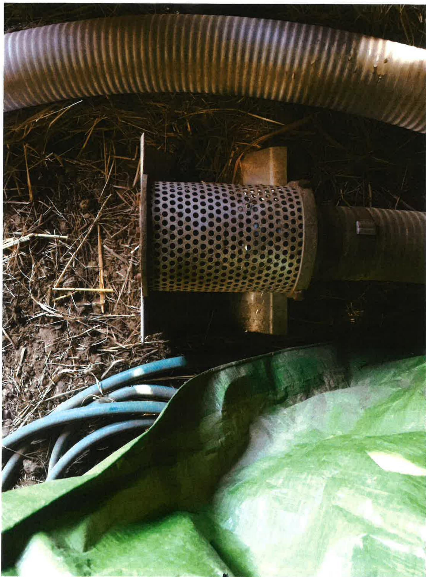
intake hose for Volume pump.
