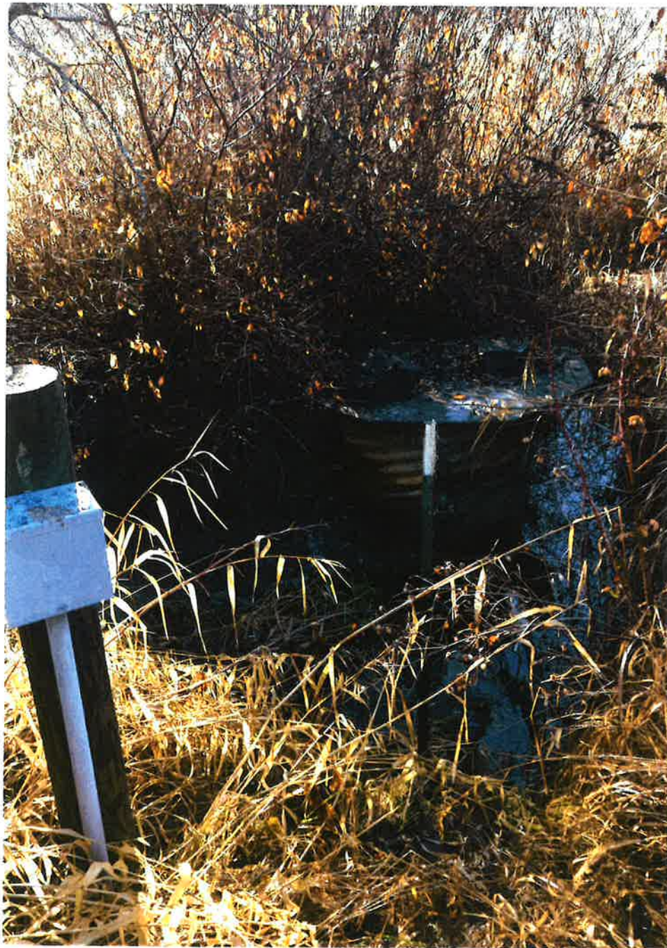
Lawn irrigation intake, electric pump
