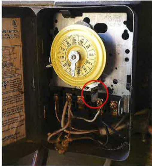
Figure 2. Pump timer On-Off switch.
