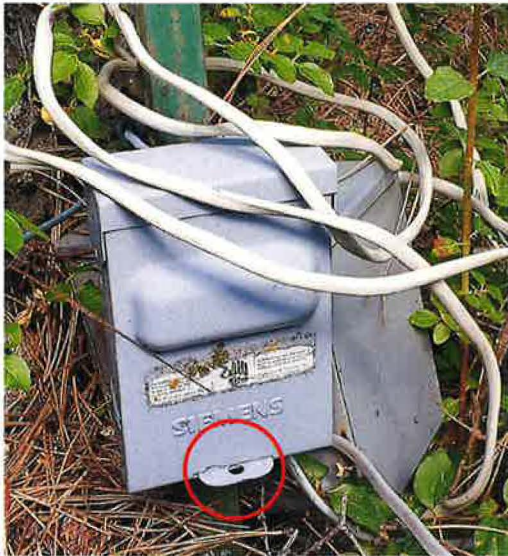
Figure 4. Circuit breaker and pump start relay.
