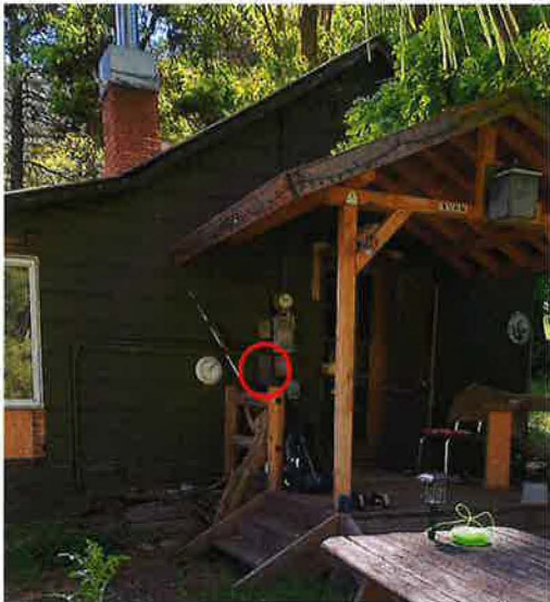
Figure 1. Water pump power supply in red circle.
