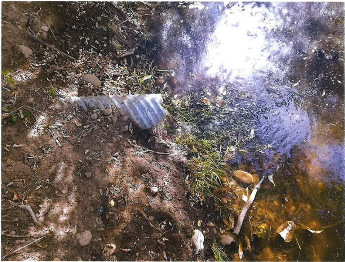
Looking at Mitigation Pipe Actively Delivering Water to the Pond (North End of Pond)
