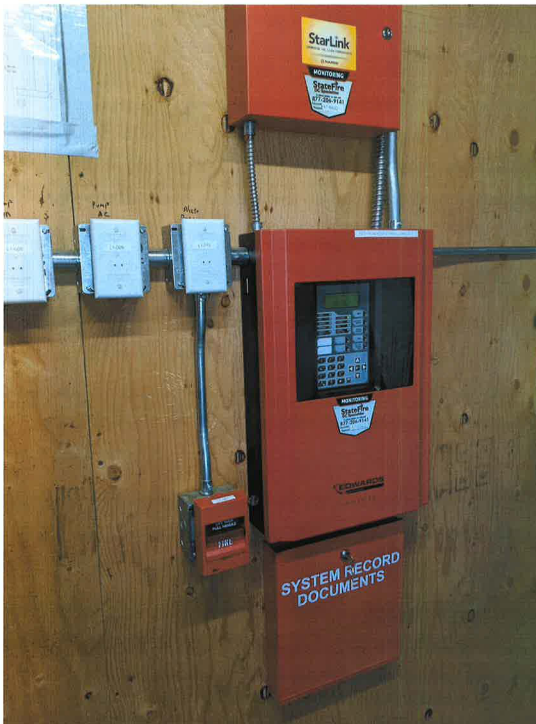
Fire Control System in Pumphouse
