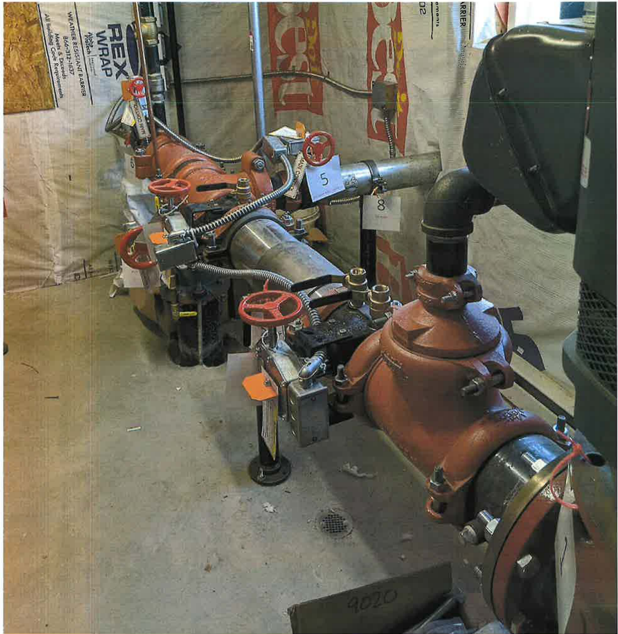
Pump House Plumbing
