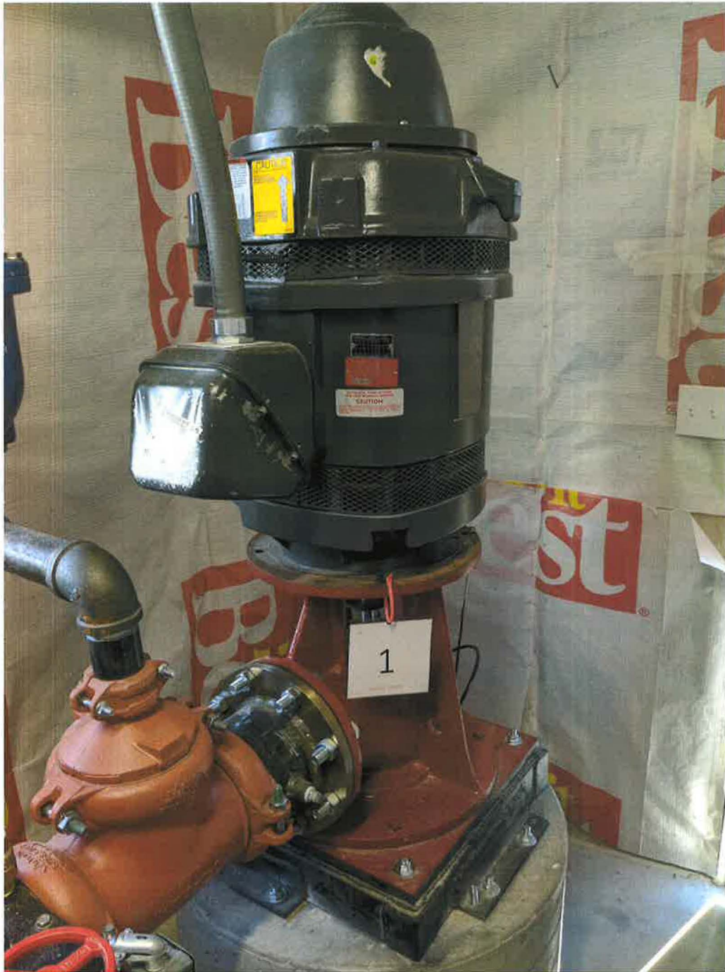
Pump Motor Mounted on Pump Drive
