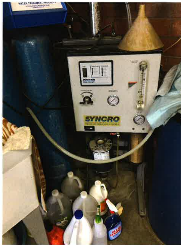
Car wash mechanical room – reverse osmosis for spot free rinse water
