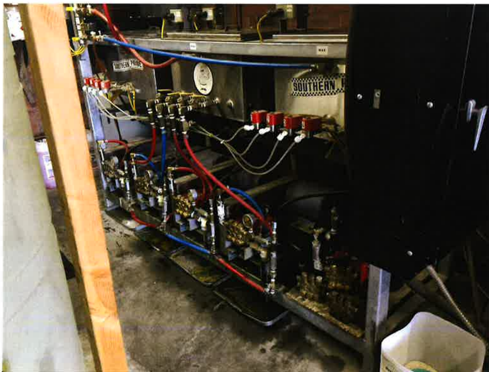
Car wash mechanical room – high-pressure pumps
