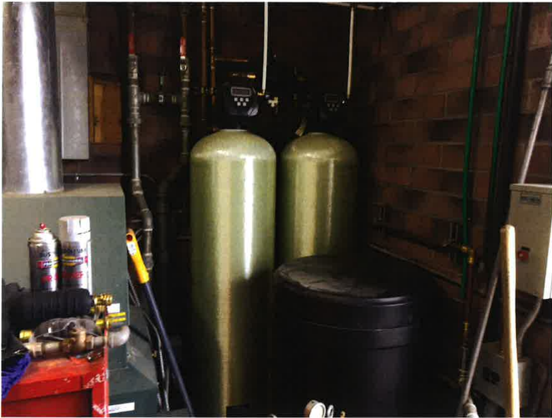
Car wash mechanical room – water softener
