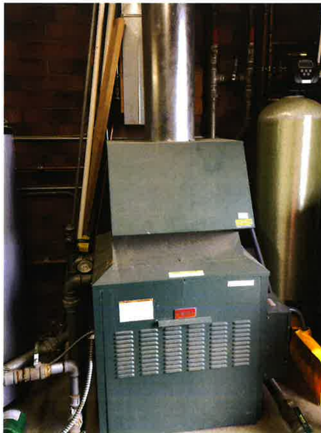
Car wash mechanical room – water heater
