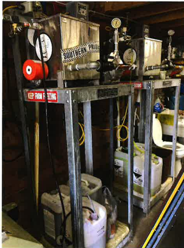
Car wash mechanical room – soap injection systems
