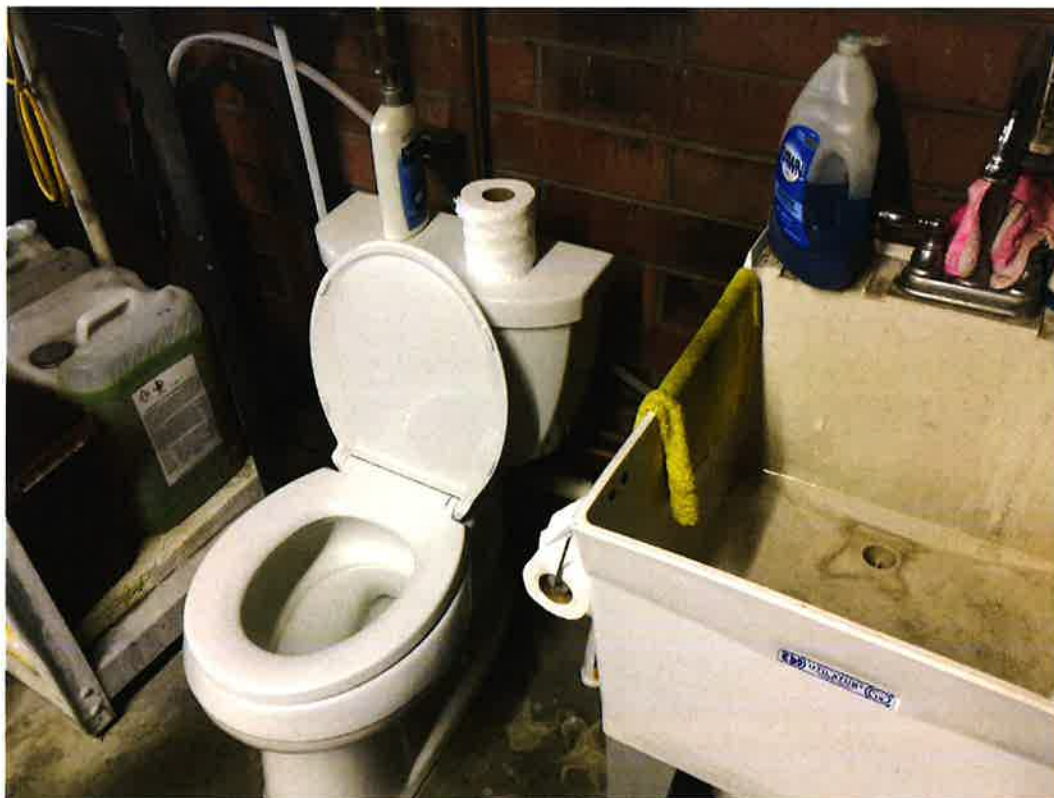
Car wash mechanical room – toilet and utility sink
