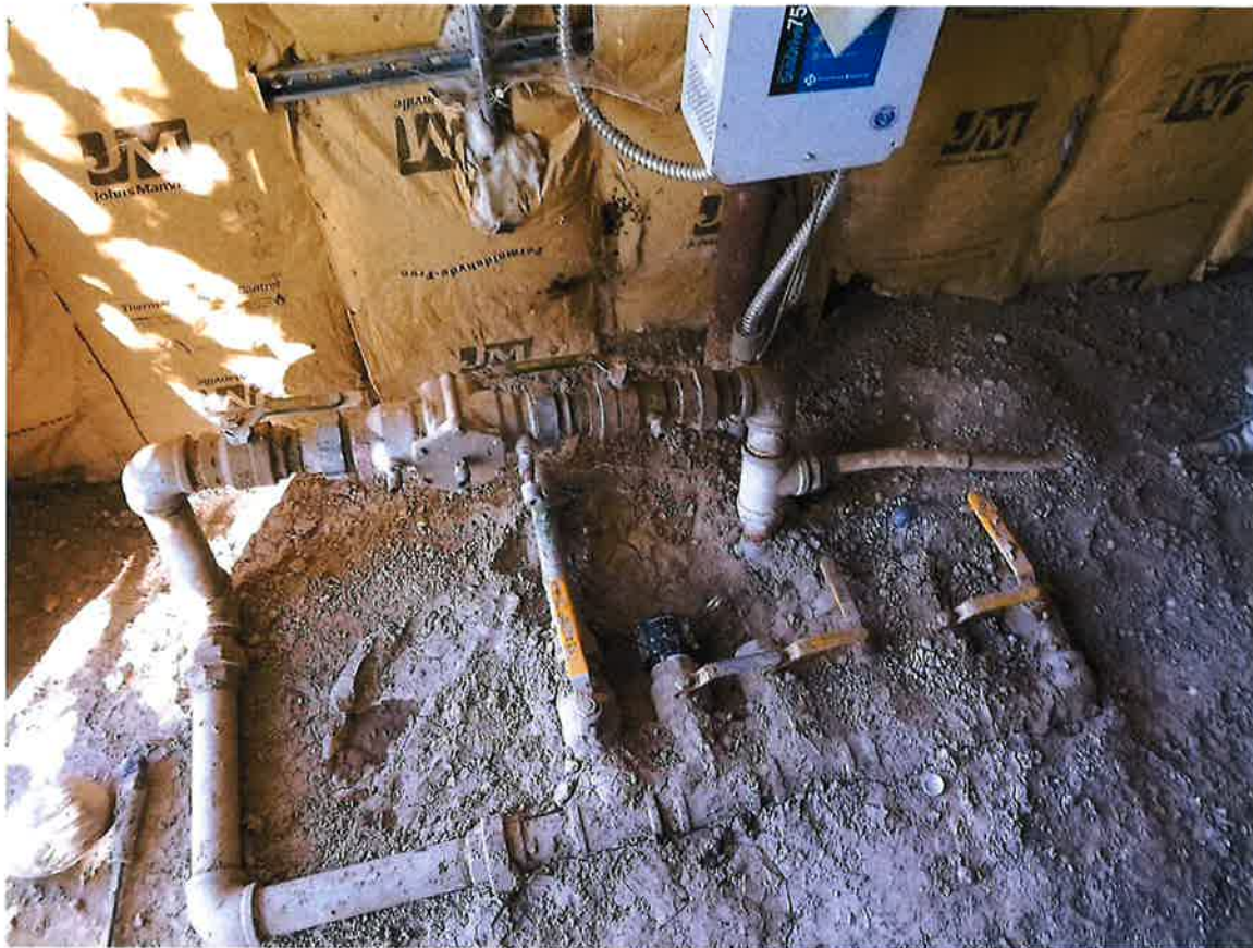
Looking at pipe configuration. 3 levers for stock and 1 lever (black coupler) for a 2 inch irrigation hose.
