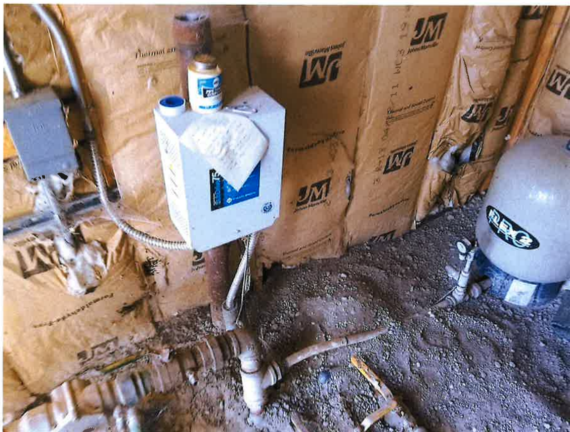
Looking at power box to submersible pump (in the well) and pressure tank inside pump house.
