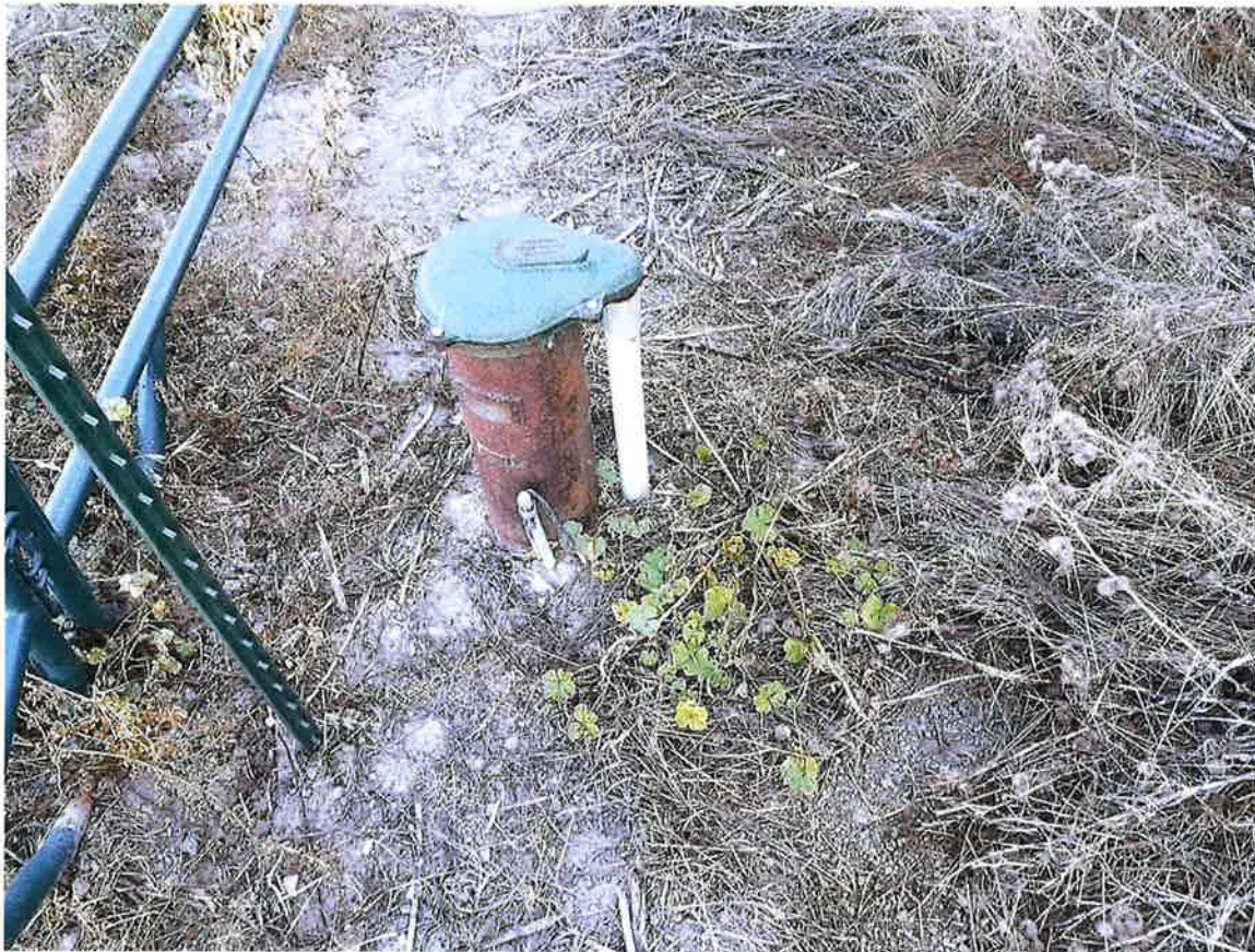
Looking at well located immediately on the west side of pump house. Well and pump house fenced off.
