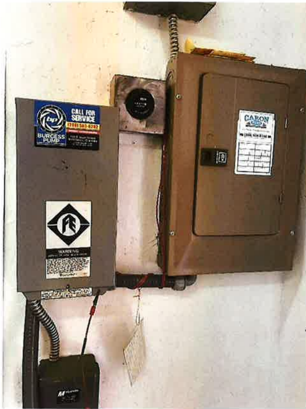
Electrical panel and meter.
