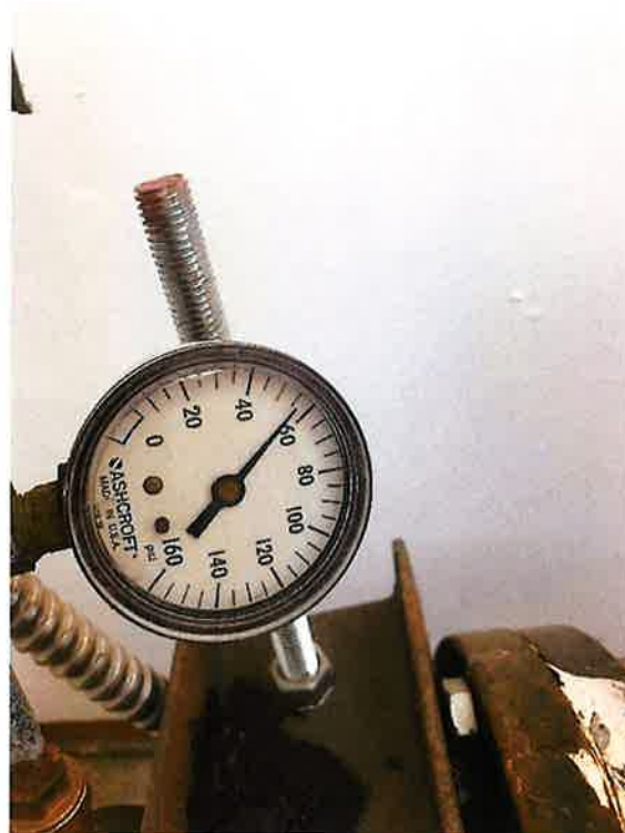
Pressure gauge prior to exit.
