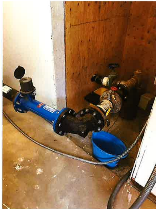
Well to the right, Totalizer meter on the left.
