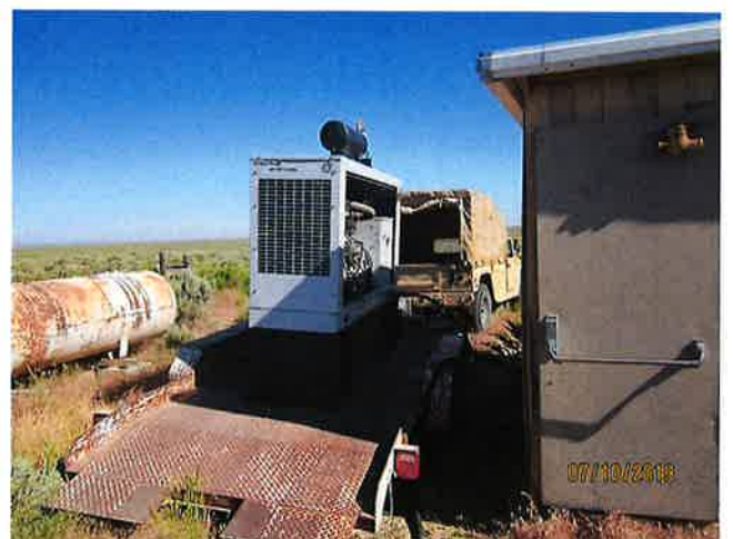
Figure 6. Portable generator used to power the pump.
