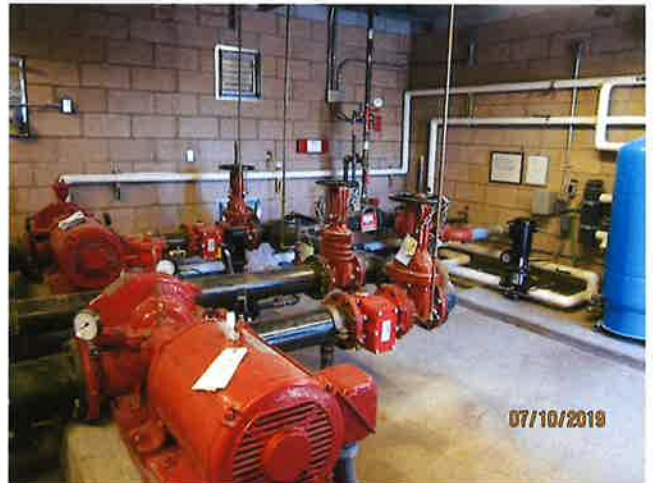
Figure 10. Panorama 3 of pump house. Large red valves and pumps are for Fire Protection under WR 51-7375.
