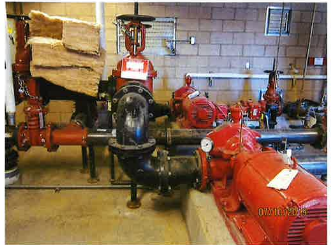
Figure 9. Panorama 2 of pump house. Large red valves and pumps are for Fire Protection under WR 51-7375.
