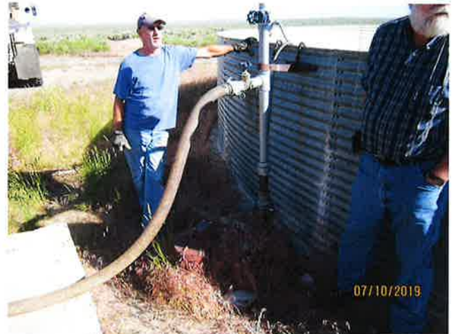
Figure 4. Pipe from the well to the hose that fills the truck.
