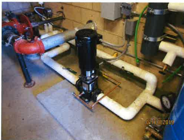
Figure 12. 2hp Grundfos pump that supplies water from the 6,000 gallon tank to the facilities for domestic and industrial use.
