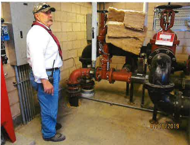
Figure 8. Panorama 1 of pump house. Large red valves and pumps are for Fire Protection under WR 51-7375.
