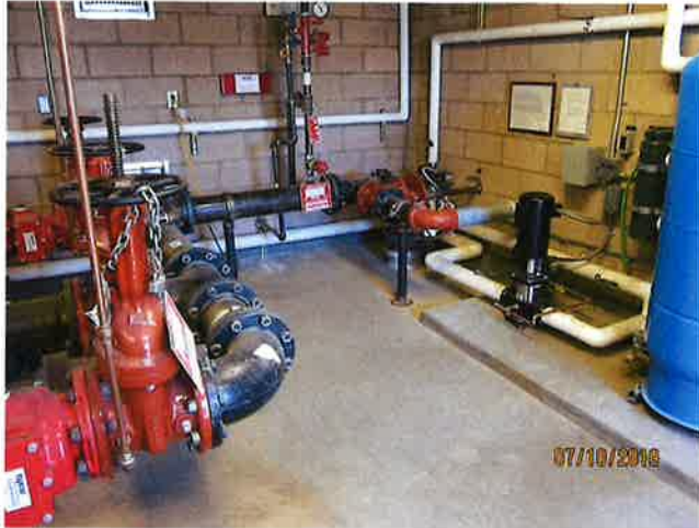
Figure 11. Panorama 4 of pump house. Large red valves and pumps are for Fire Protection under WR 51-7375. Black pump in right side of the picture is the 2 hp pump that services the domestic/industrial for this permit.
