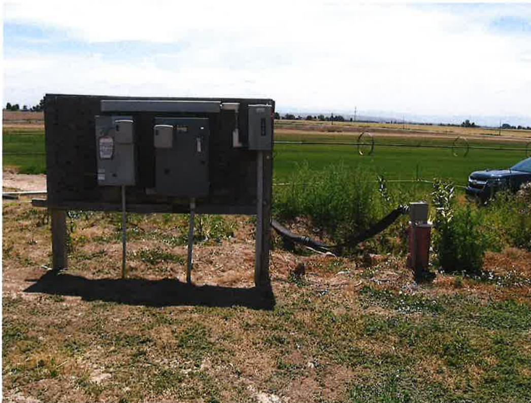
The pump control panel with the Groundwater POD shown to the right. The holding pond is to the left of the photograph.
