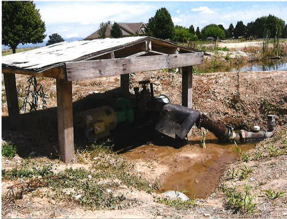
(Above) Surface Water Pump which draws water from the holding pond seen in the upper right corner of the picture. The Farr Lateral which gravity feeds water into the holding pond is just beyond the dirt access road behind the pond.
