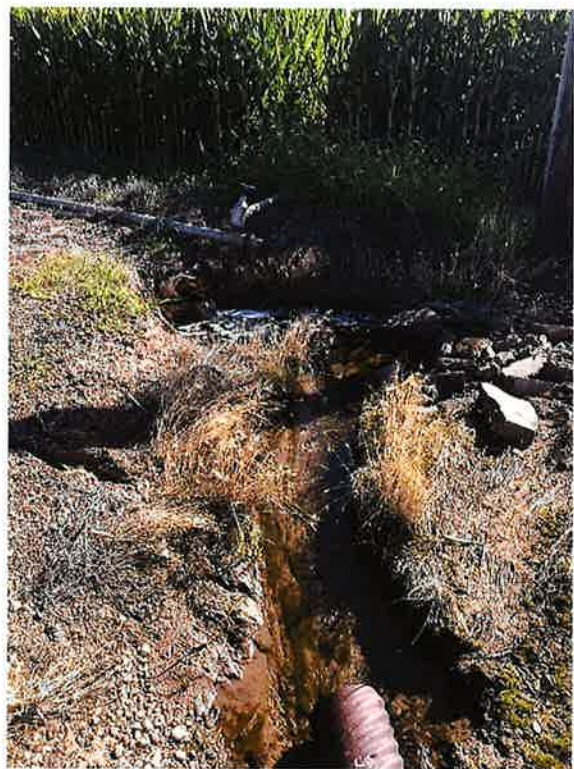
Waste water drainage.
