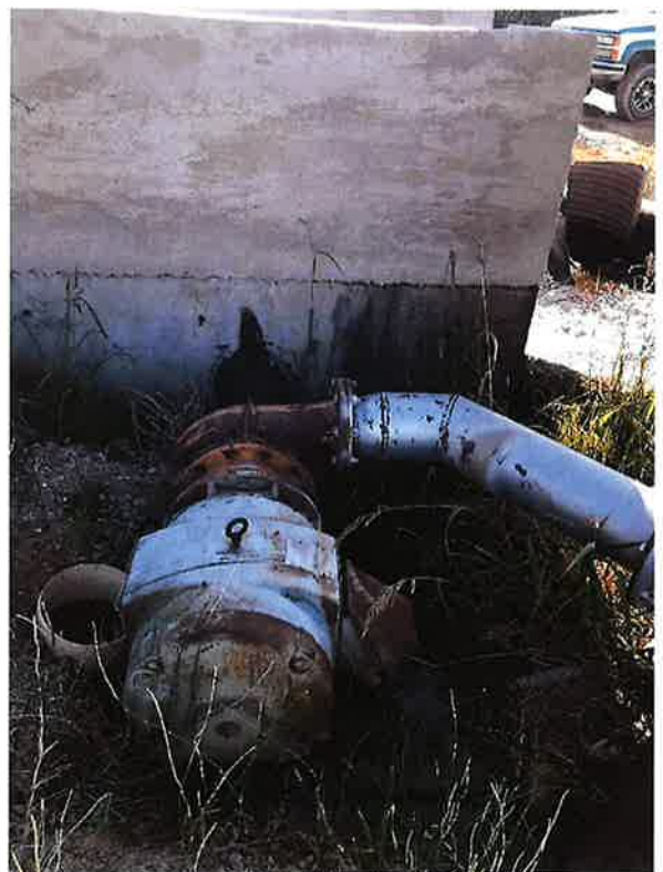
Pump for the large pivot.
