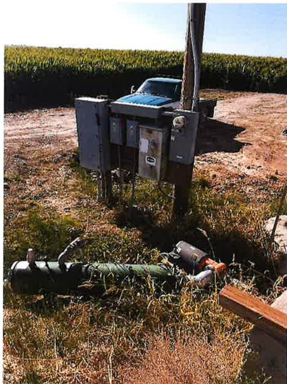
Power board for well and pump to small pivots.
