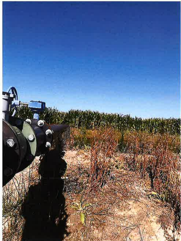
Valves and meter on well.
