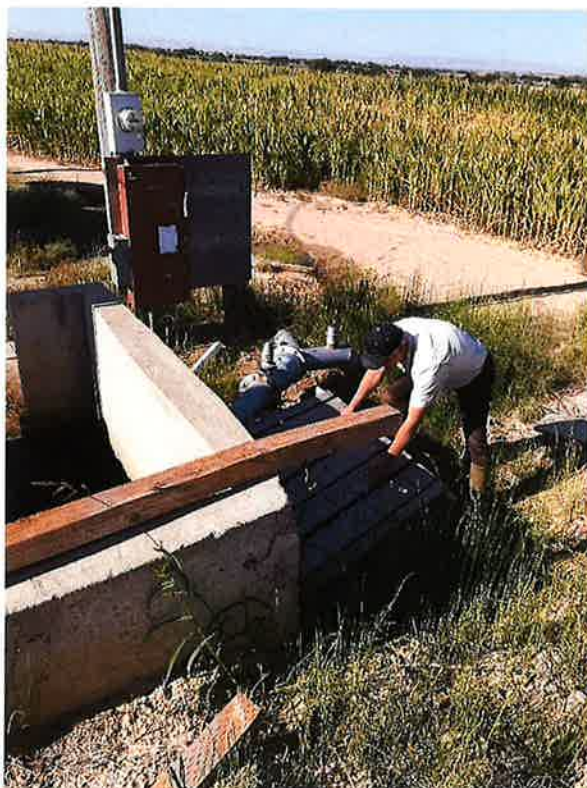
Photo of pump for the large pivot taken from the edge of pond. Power board for this pump.
