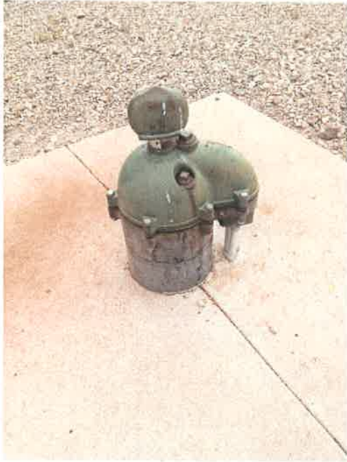
Figure 1 The 12" well with one 75-hp pump used to supply water for domestic and irrigation purposes.
