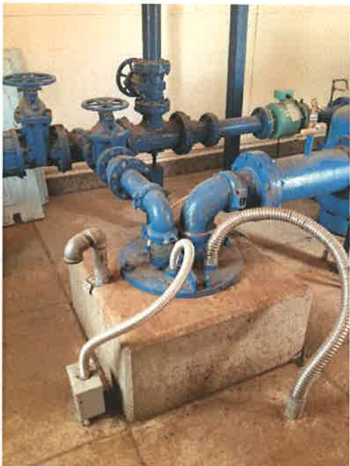
Figure 2 The 18" well with a 30-hp pump for domestic and irrigation uses and a 125-hp pump used for fire protection.
