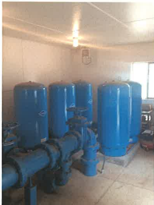
Figure 4 5 pressure tanks used as part of the domestic/irrigation system.
