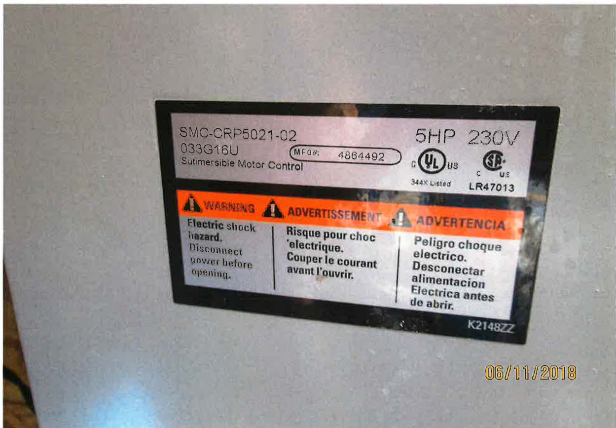
5hp pump in well.
