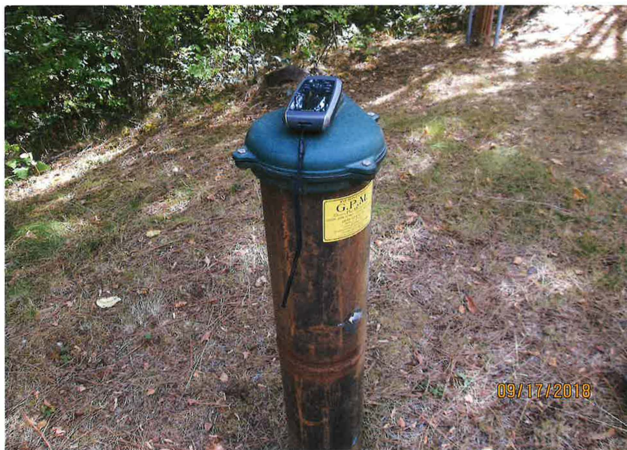
Well D0040419 with 5hp pump.
