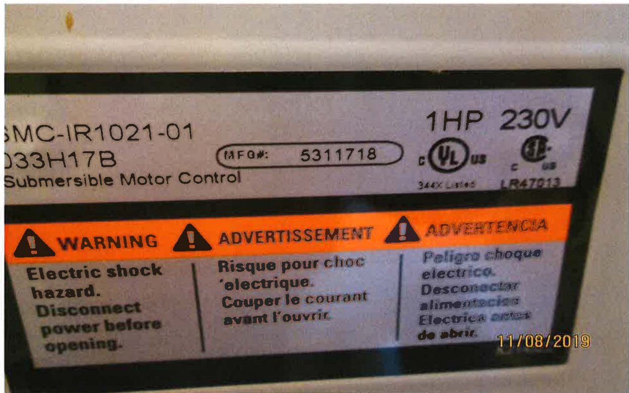
1 hp pump in well to 1,500 gallon storage tank.
