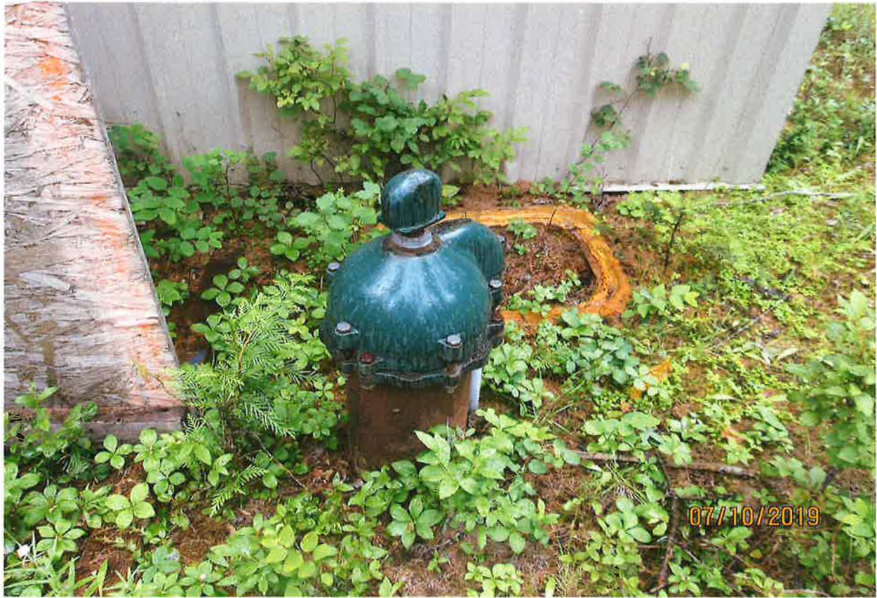
Well 2, log 97-96-N-0046. 10hp pump.
