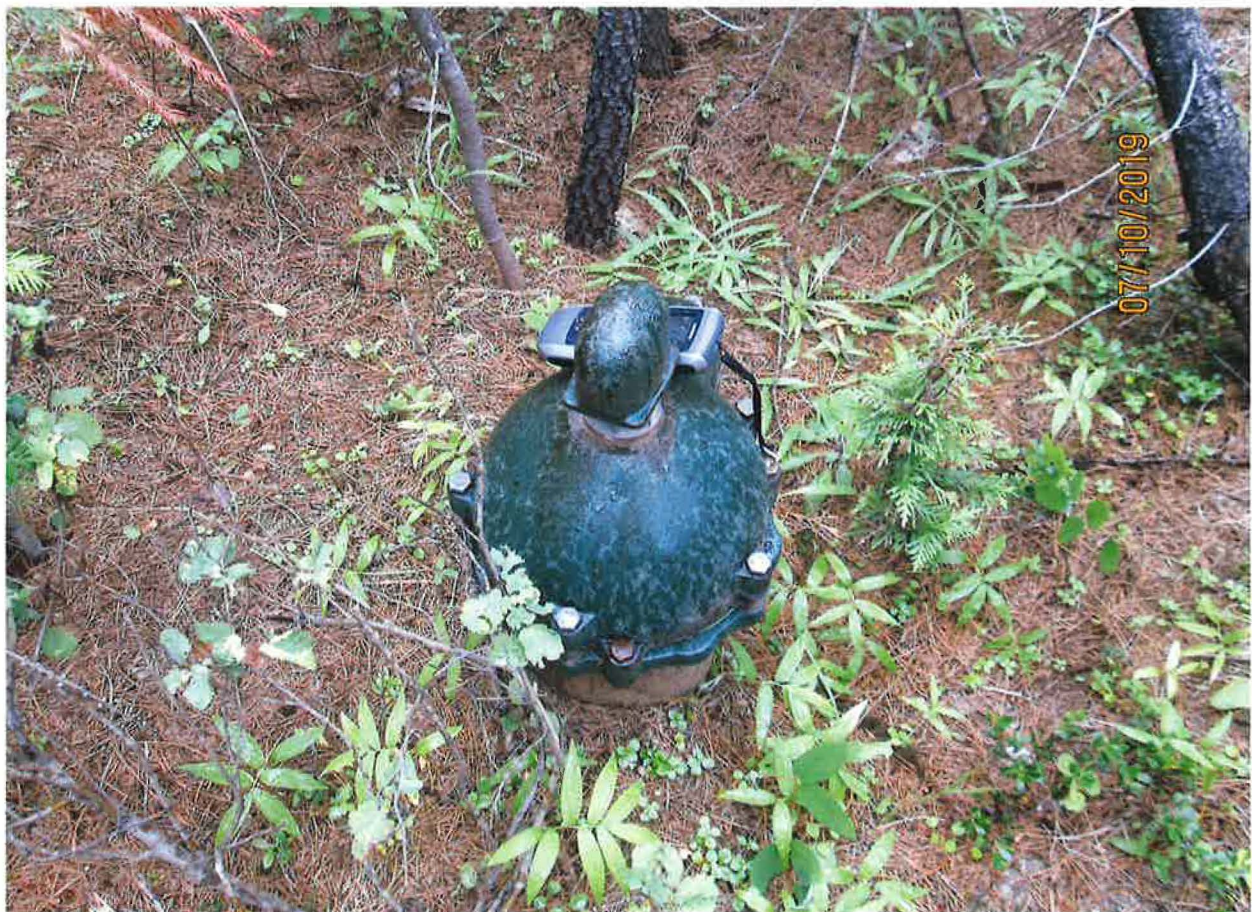
Well 1, log 97-96-N0001. 10hp pump.
