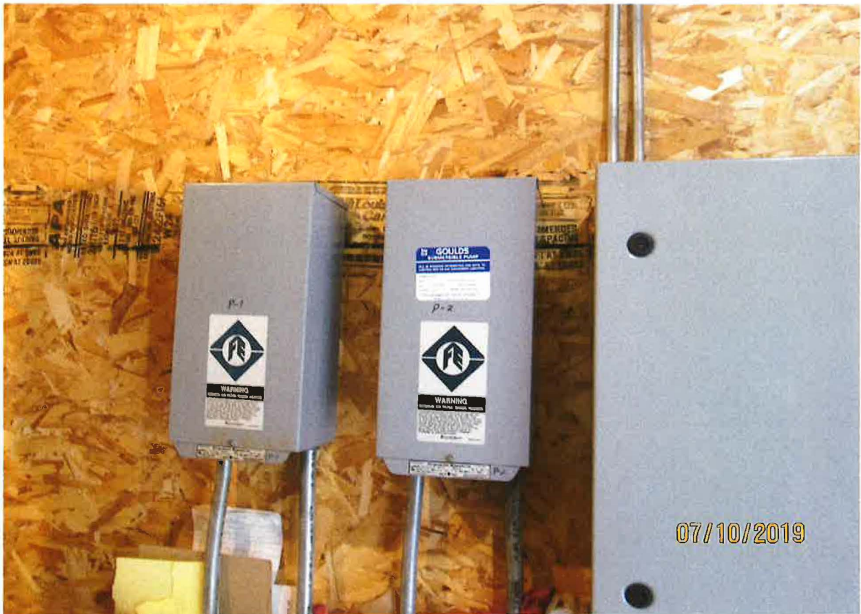
10hp pump electrical boxes.
