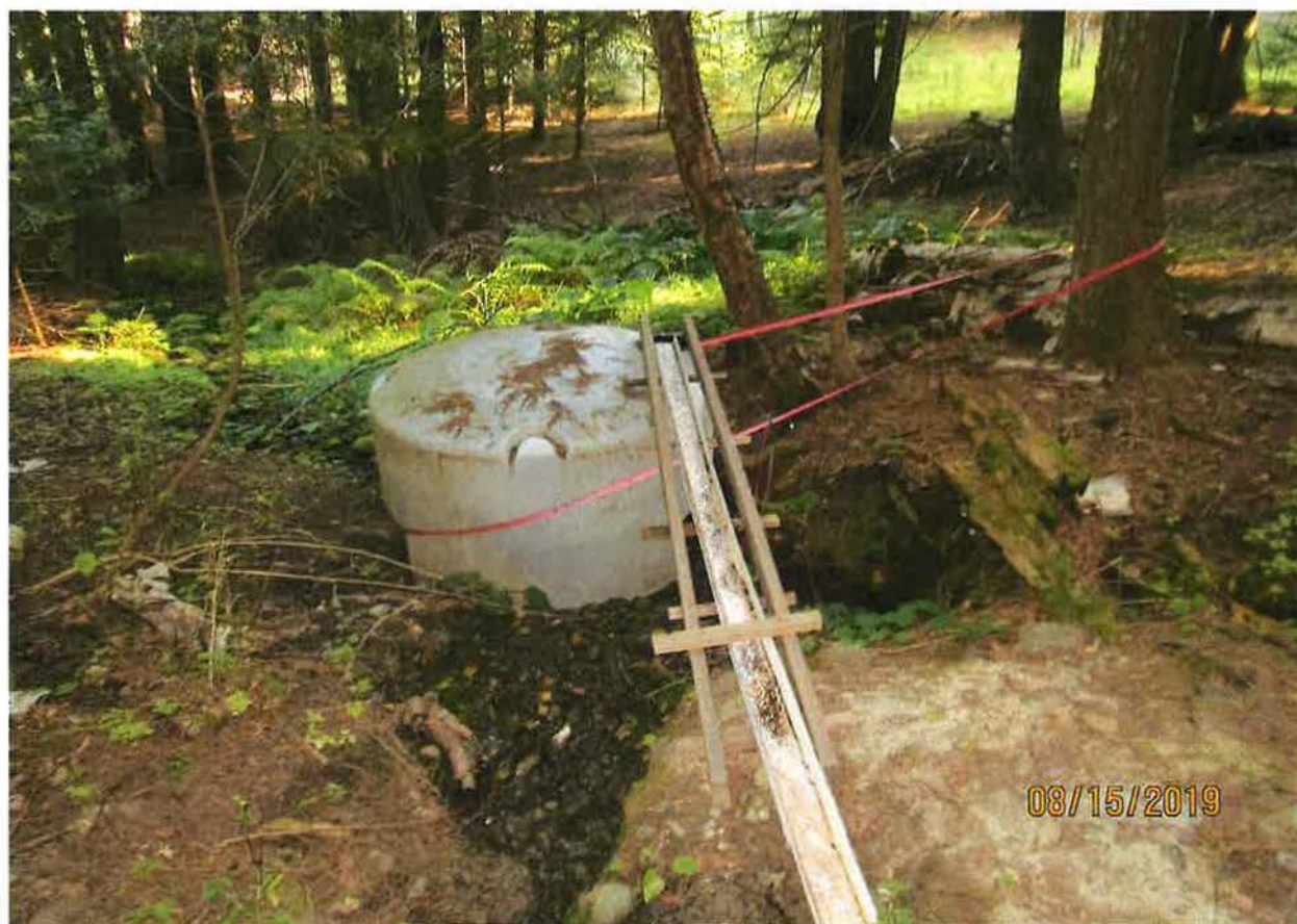
Diversion from spring to 500 gallon storage tank.
