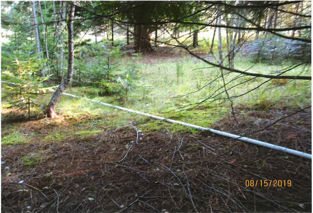
2 inch pipeline used for gravity flow to irrigation.
