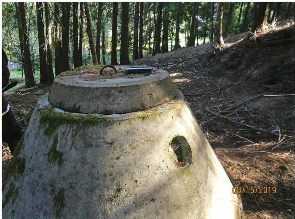
Spring POD. System was gravity fed to home.
