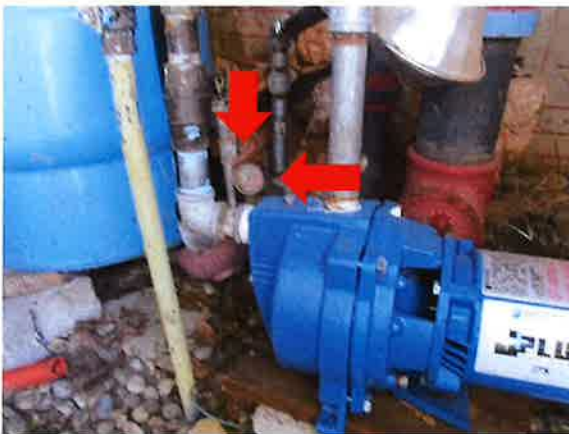
Pressure gage between pump and pressure tank.
