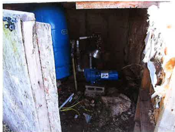
Well, pump and pressure tank
