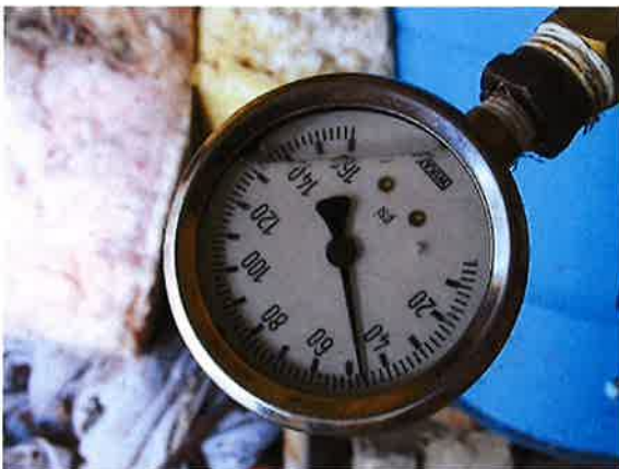
Pressure tank with pump running = 46 psi
