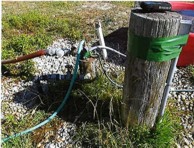
Well and hose distribution system.
