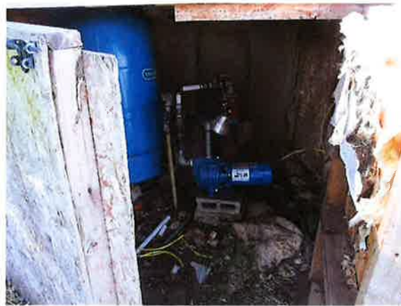
Well, pump and pressure tank
