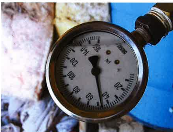
Pressure tank with pump running = 46 psi
