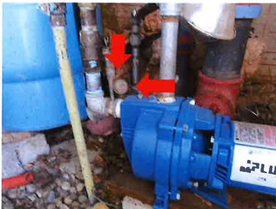
Pressure gage between pump and pressure tank.
