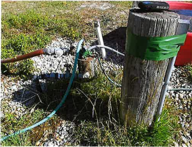
Well and hose distribution system.
