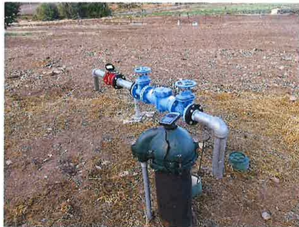
Photo #1 – Well and Flow Meter
