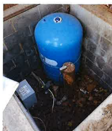
Corral Well (Well #3) with associated pressure tank and supply line with pressure gauge (reading 53 psi while on site).
