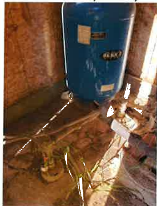
Weigh Station Well (Well #1) and associated pressure tank.
