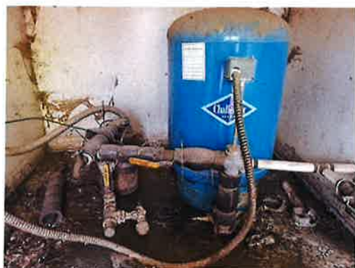
Barn Well (Well #4) and associated pressure tank.
