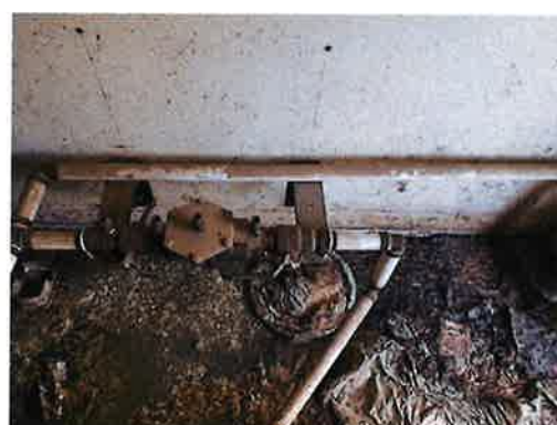
Barn Well (Well #4) supply line.
