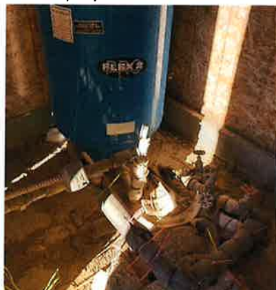
Weigh Station Well (Well #1) supply line.
