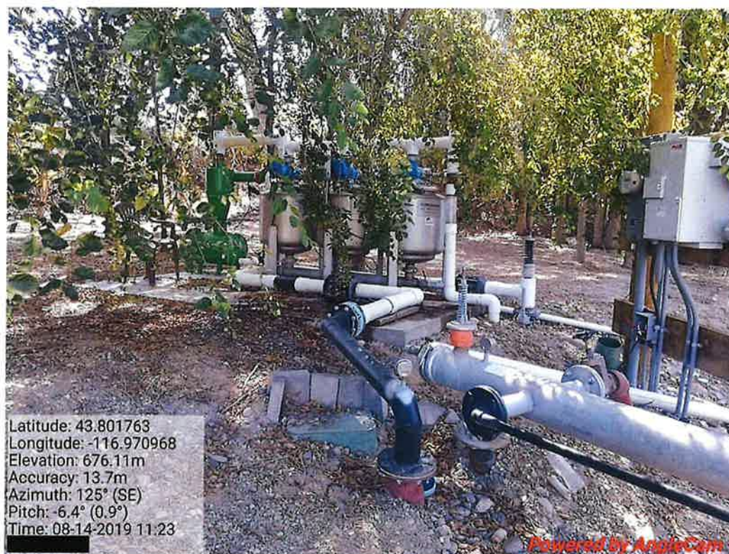
POD 935524: Filtration system for lawn sprinklers. Motor and pump are to the right.
