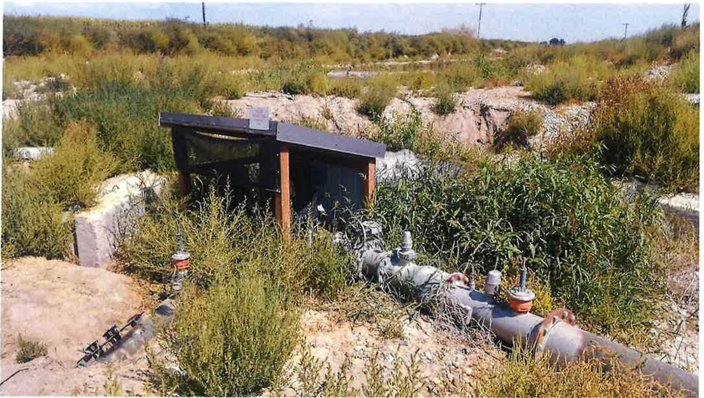
POD 935523: Unnamed drain is seen at the top of the picture. Bubbler is behind the motor covering. The left pipe is the 8 inch pipe supplying the western pivot. The right pipe supplies the eastern pivot and hand lines.
