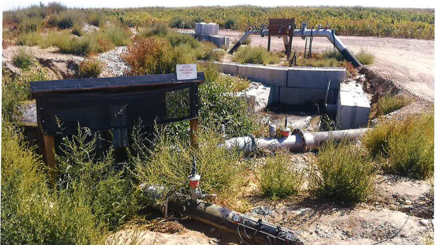
Same as the above photo looking towards the SE. Drain continues under the road to the right.
