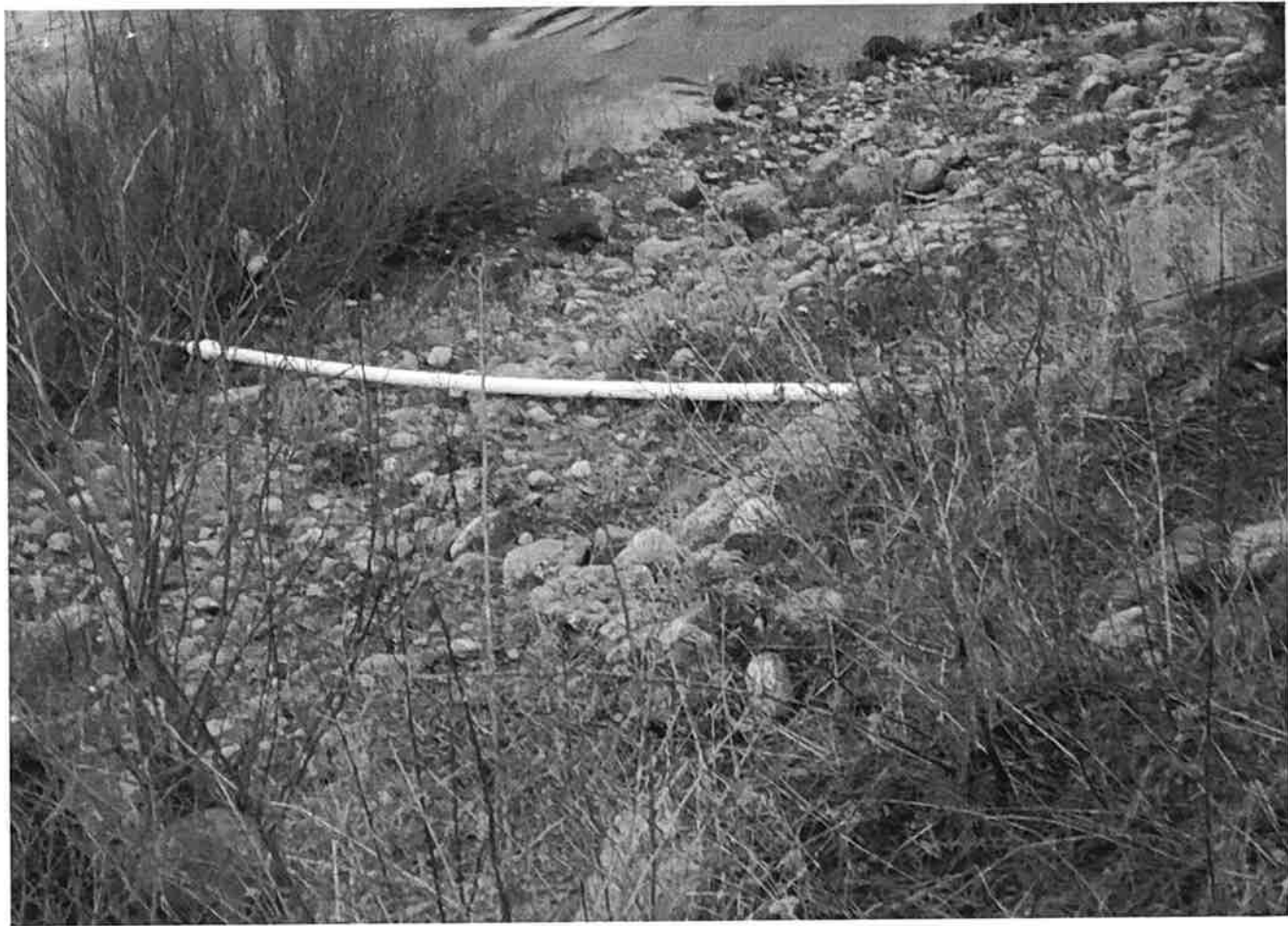
Pipe up from River to Pump
