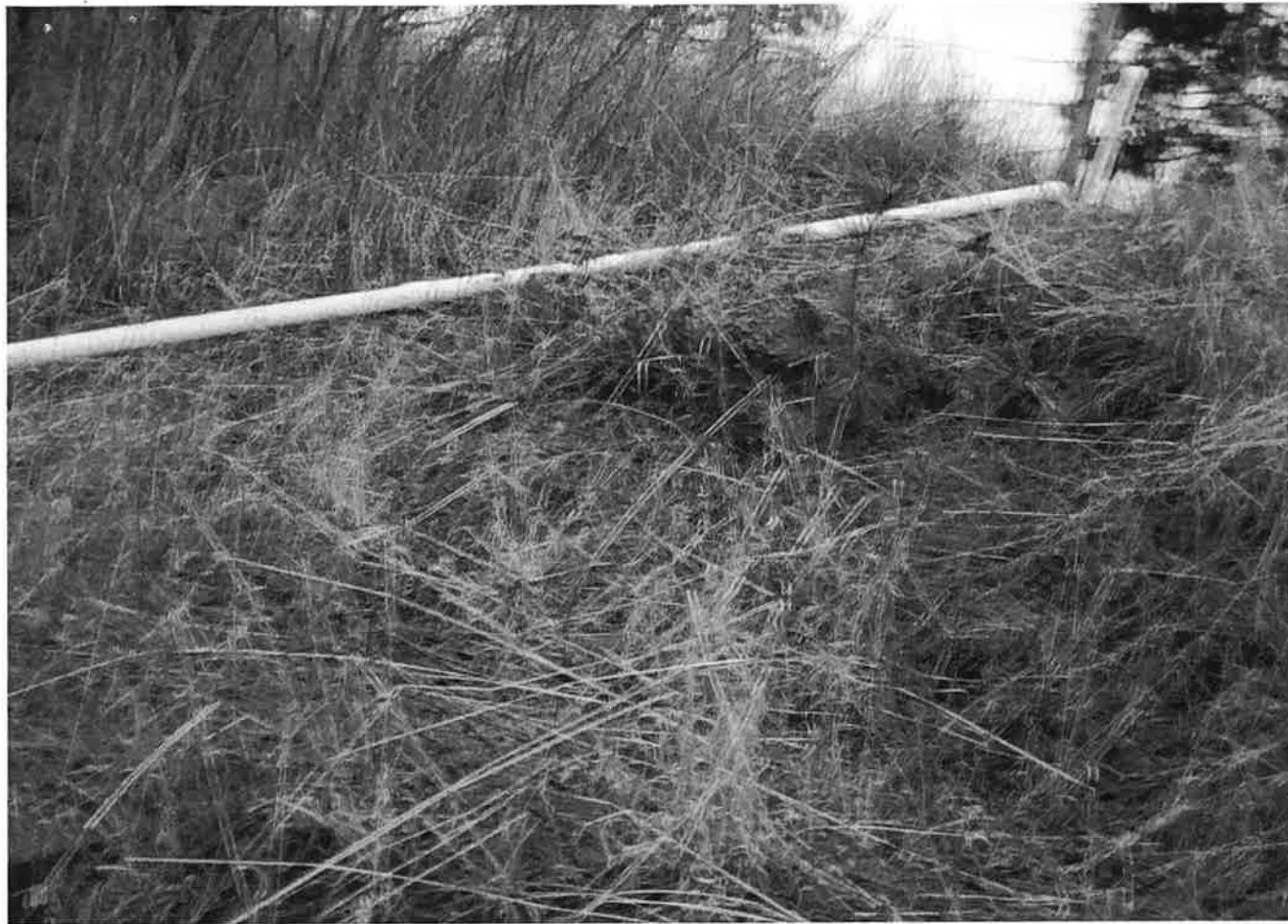
Pipe From Pump up to spicket
