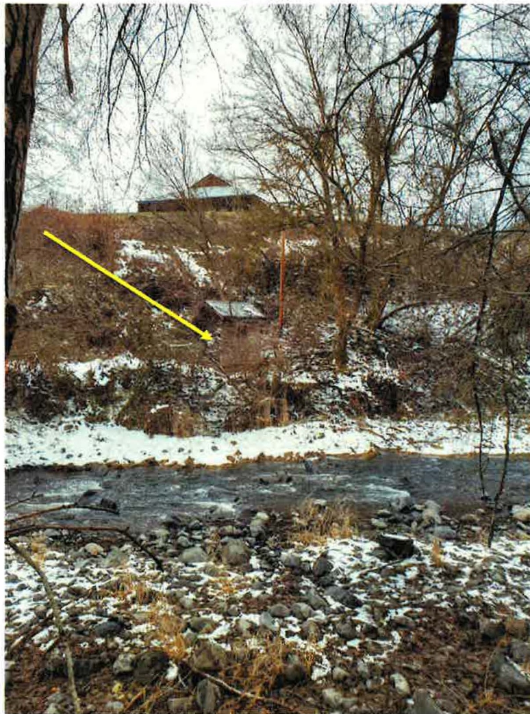
Figure 2. Picture of old abandoned pumphouse structure where pump and piping used to be for withdrawing water (Point of Diversion) to irrigate the farm (water rights 85-2118A, 85-2118B, 85-2118C, 85-15799, 85-15800, 85-4214). Renberg barn in background.
