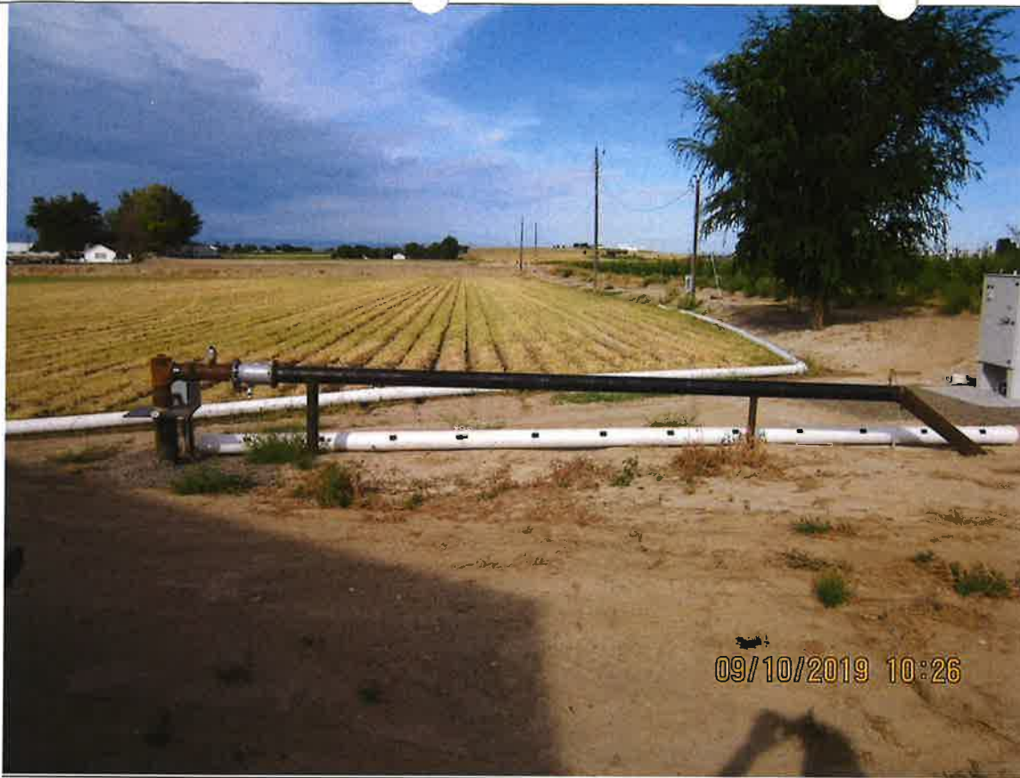
Figure 3. Outlet pipe extends over another underground pipeline.
