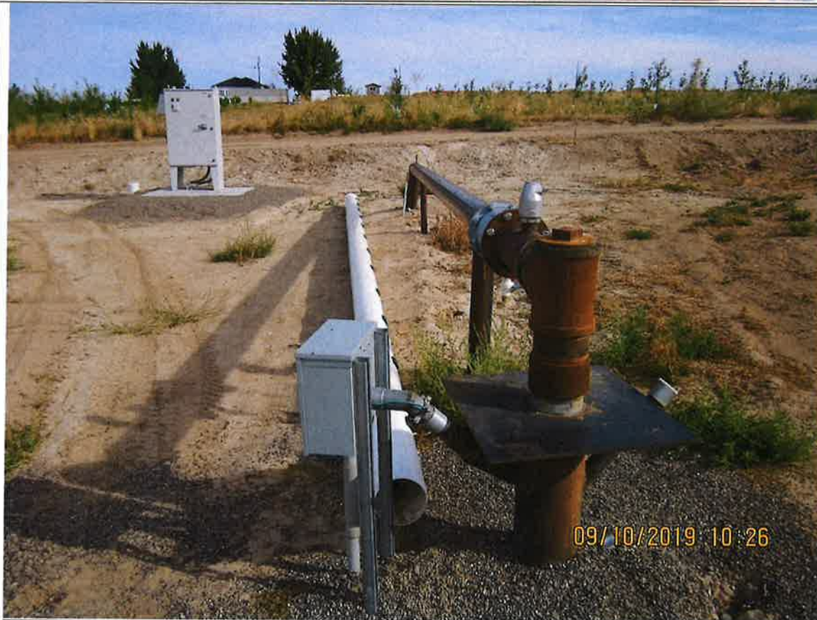
Figure 2. Well head and control panel.
