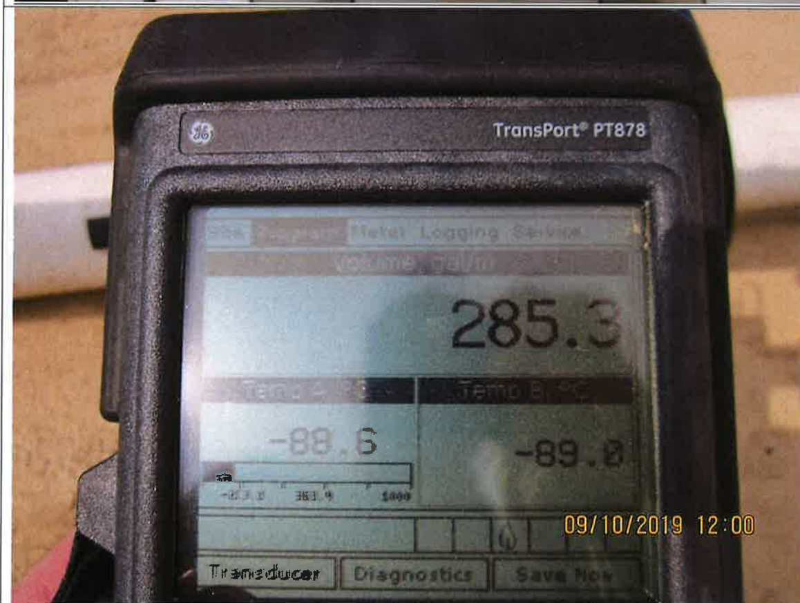
Figure 6. The first Panametric flow meter measurement taken along steel pipe was 285.4 gpm or 0.64 cfs.
