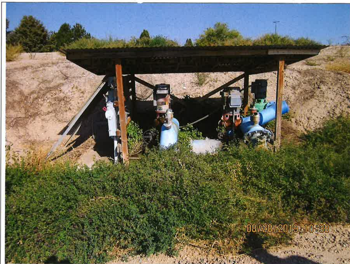
Figure 7. Pumping station from pond.
