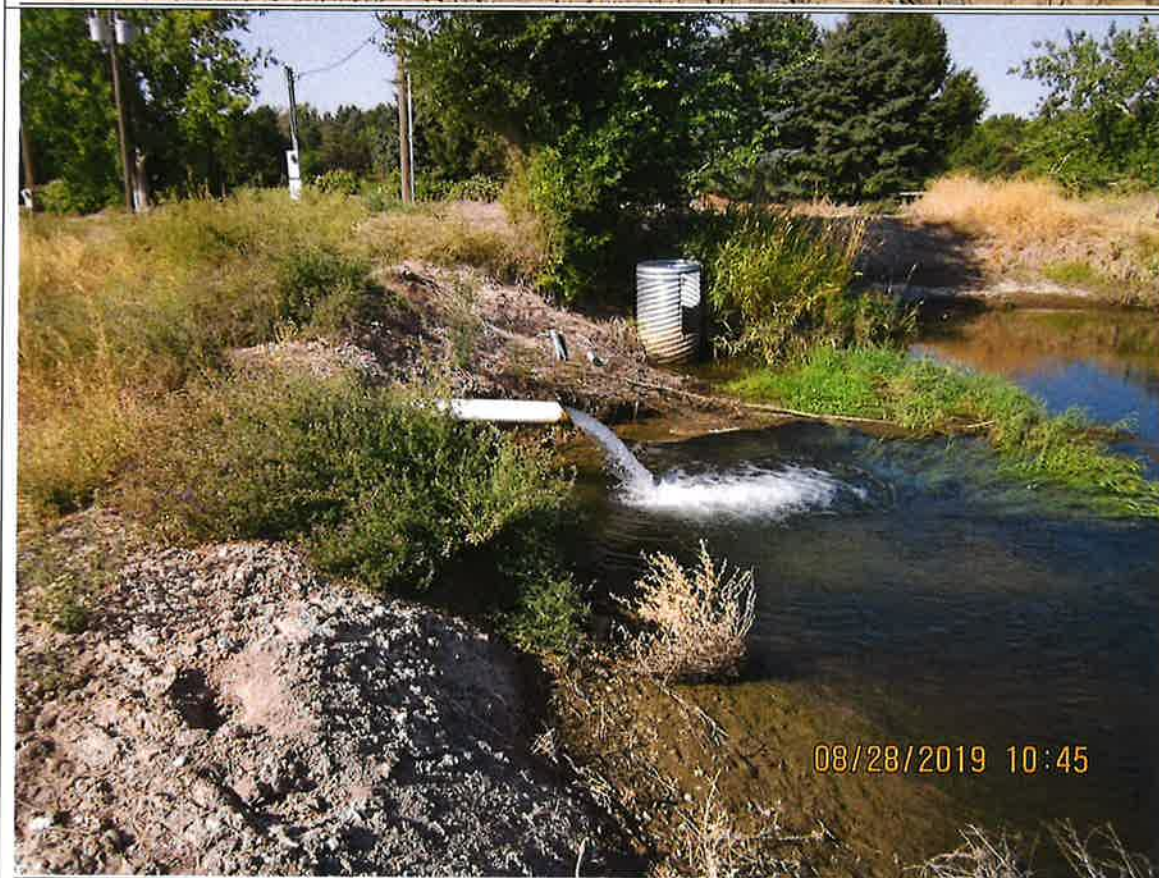
Figure 2. Plastic outlet pipe goes through bank and open discharges into pond.
