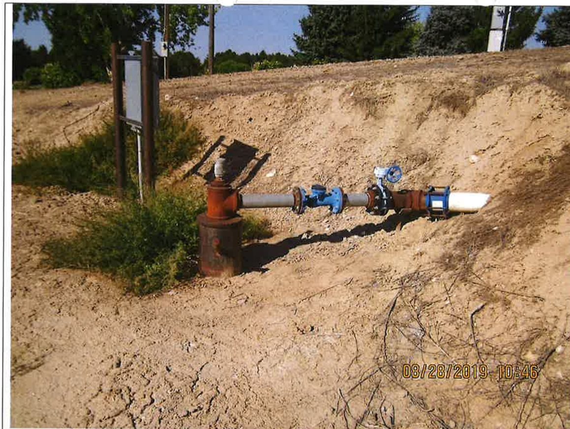
Figure 1. A 14-inch well casing goes to a 4.5 inch galvanize pipe through a flowmeter and valve to an 8-inch plastic outlet pipe.
