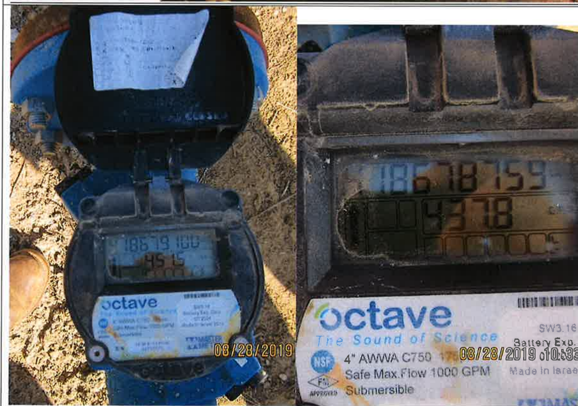
Figure 4. Master Meter Octave flow meter, readings varied from 437.8 to 451.5 gpm.
