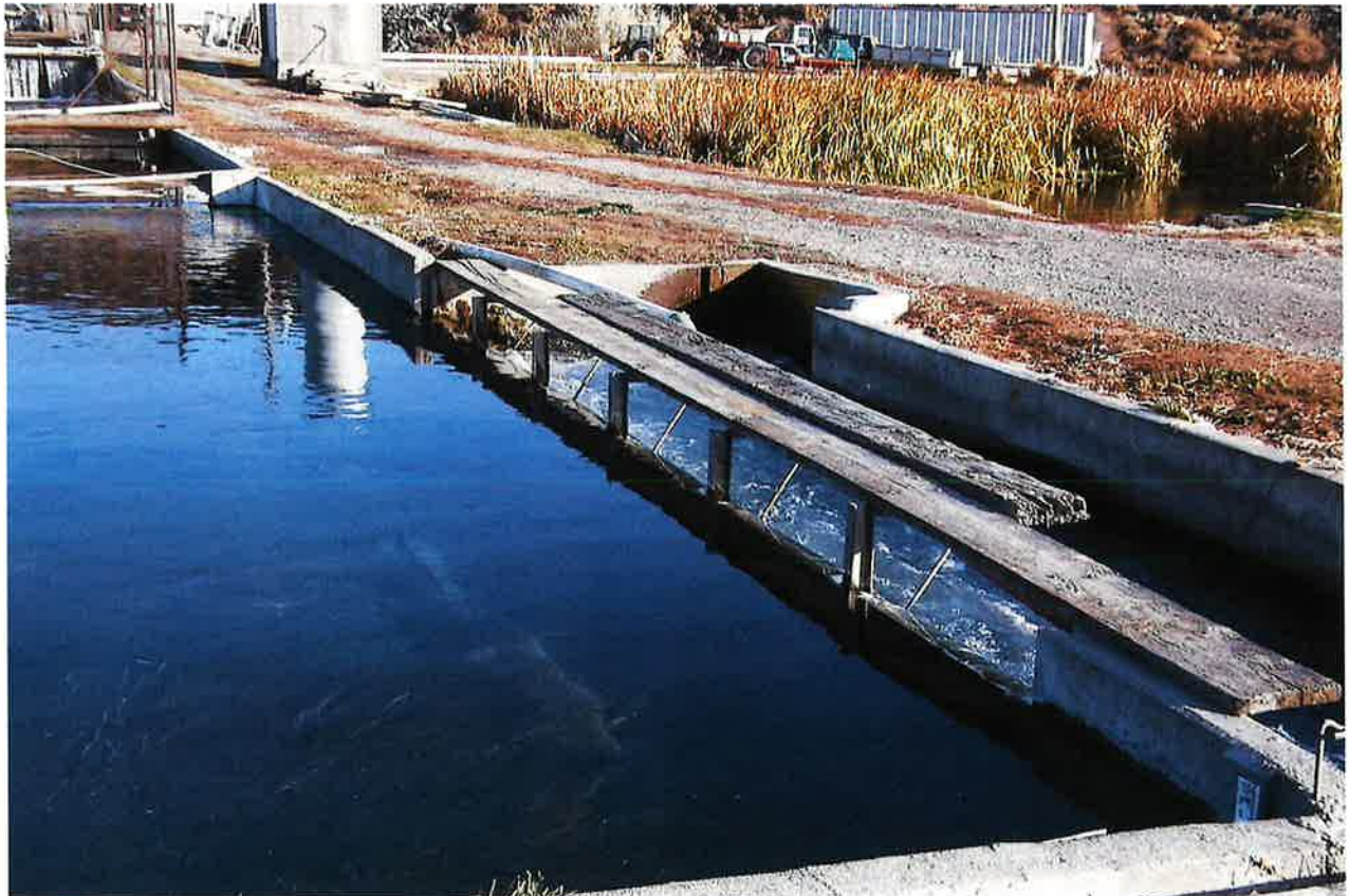
The exit weirs at the outlet of the fish facility.
